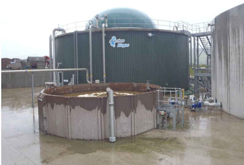
Liquid feed tank and digestate storage tank
