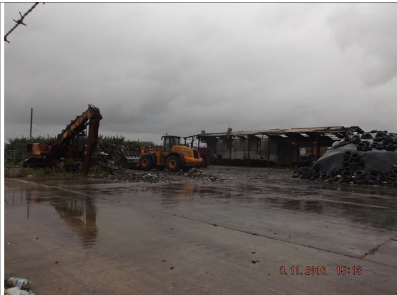
Waste has started to be removed from the fire damaged waste pile
