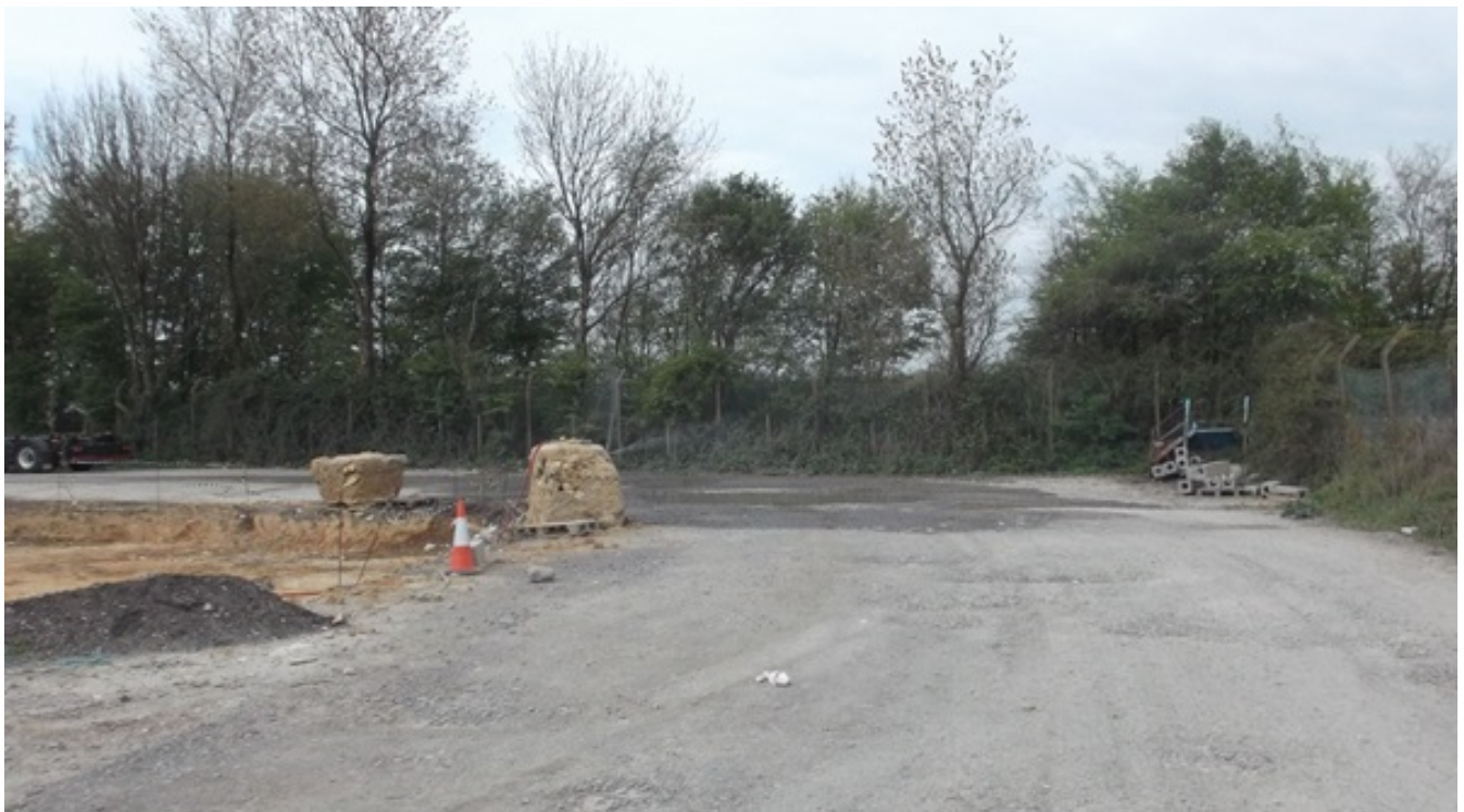
Siteserv's track at the rear of Hangar A; road is currently dusty and full of pot holes. This road is due to be tarmacked.
