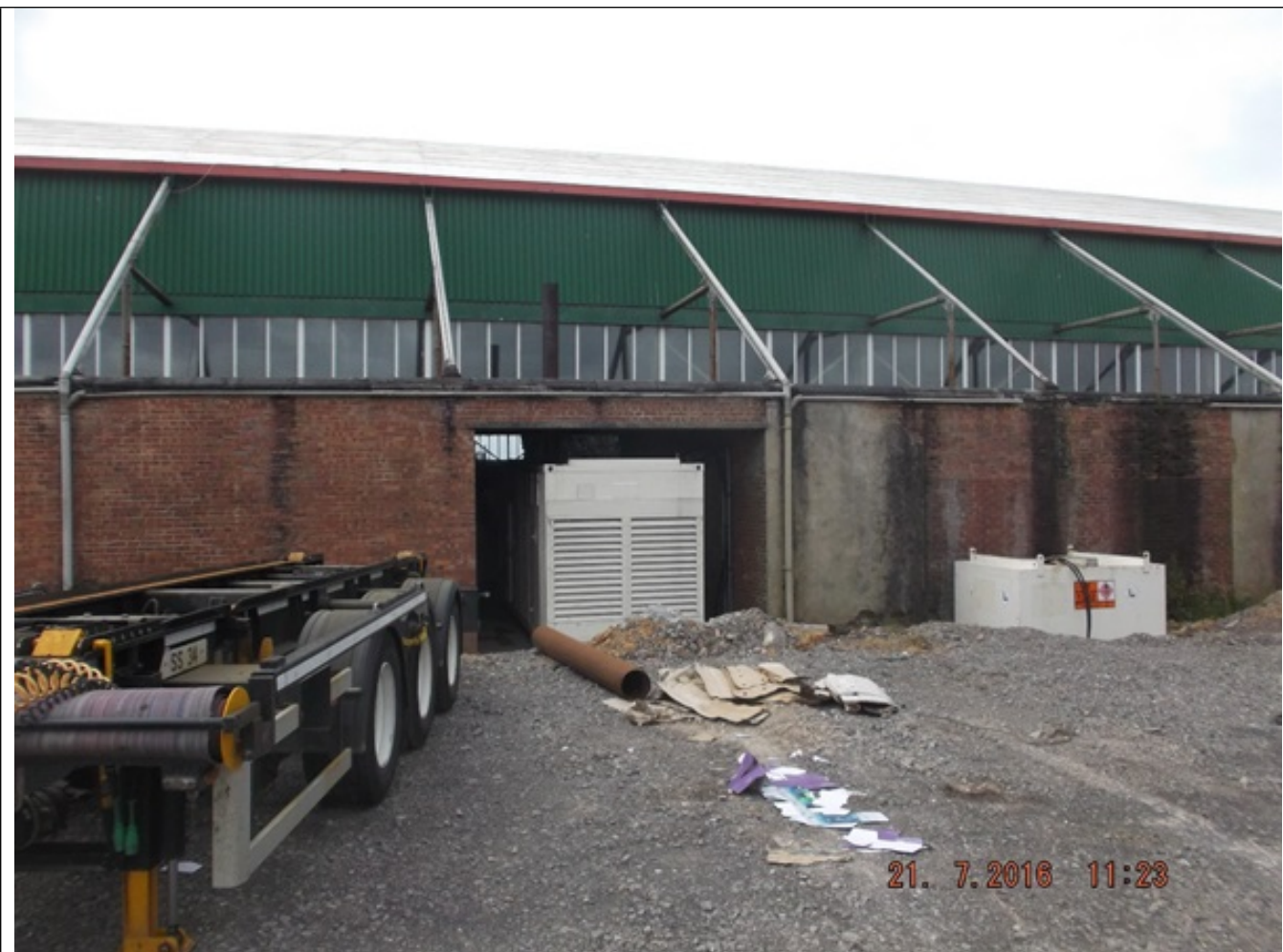
The generator, now contained within an alcove of Hangar A
