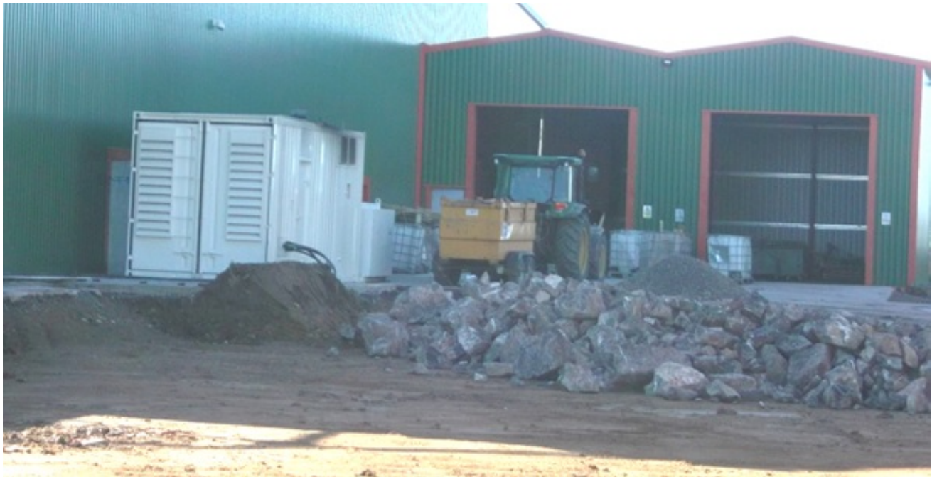
Generator and biomass boiler at the back of hangar A
