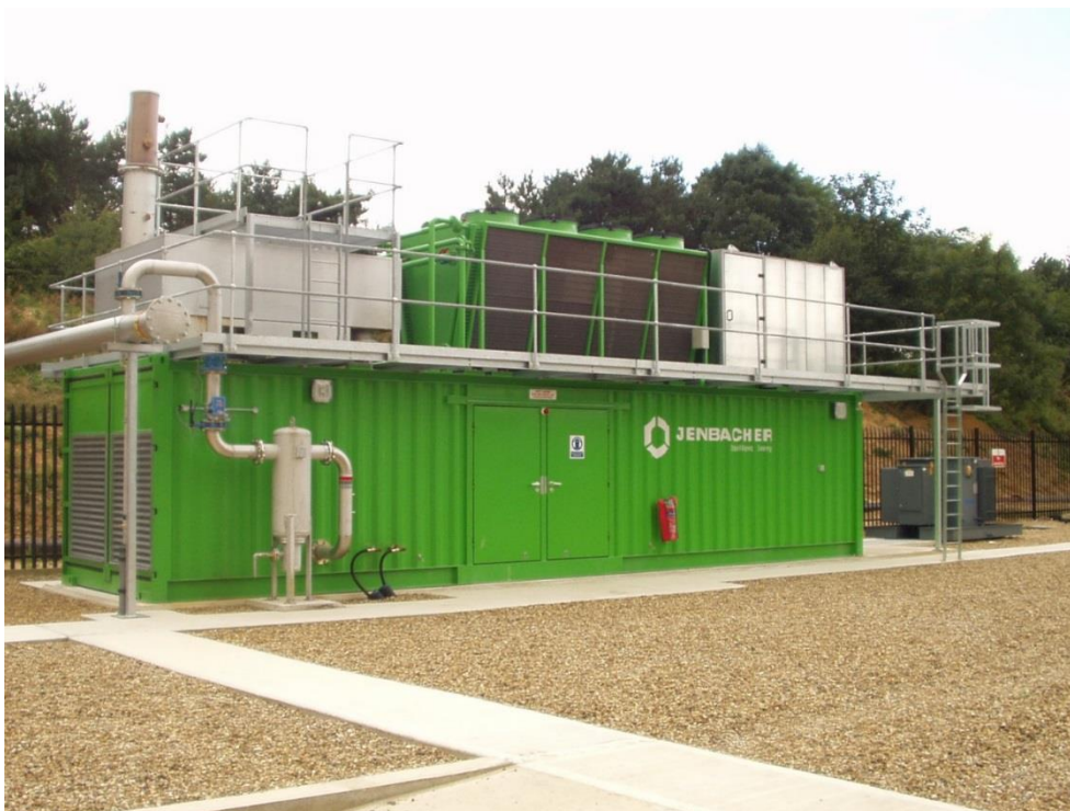
Figure 3.2 Photograph of the Proposed Engine Generating Set
