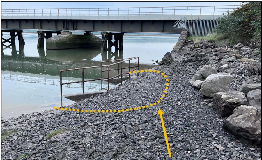
Figure 5: Machine movement area behind tidal flap.
