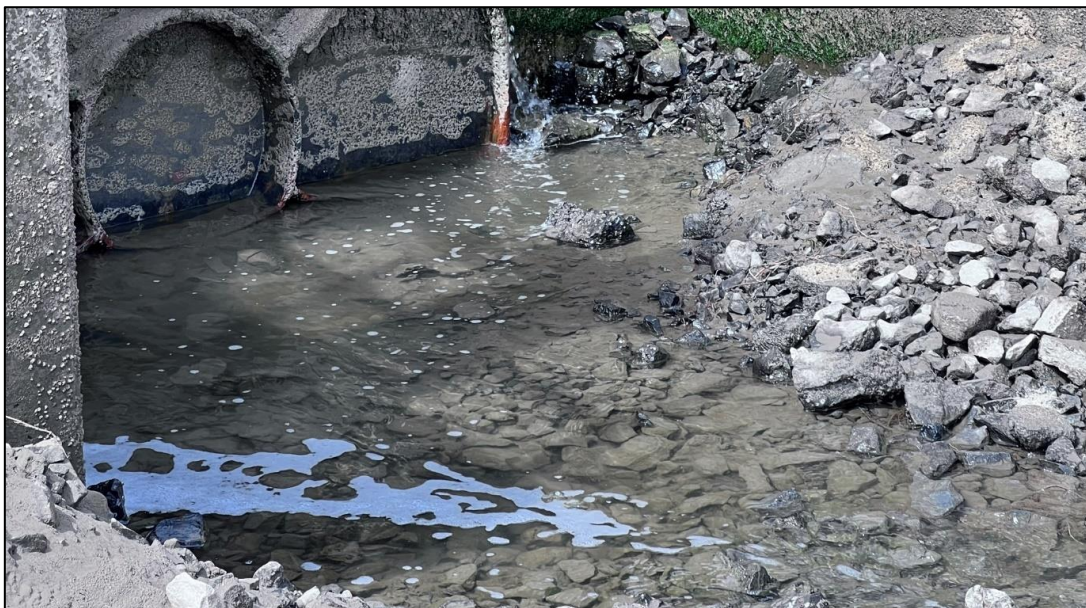
Figure 2: Blocked tidal flap.
