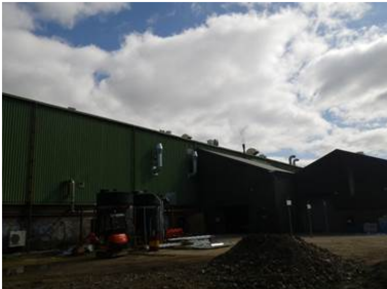
Photo 12: New extraction vents
