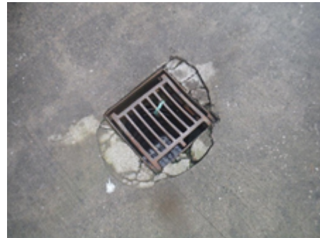
Photo 2 – Cracks around drain in ETP bund
