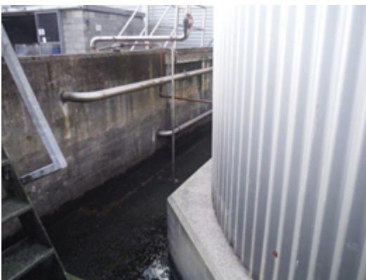
Photo 4 – Pipes penetrating the bund wall
