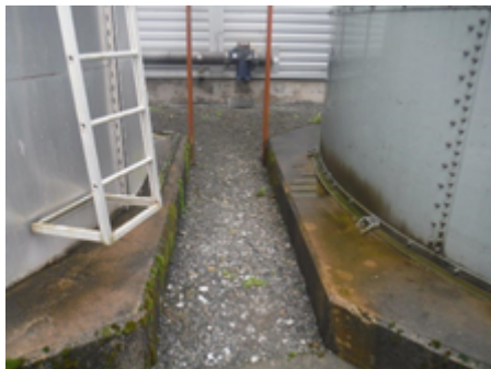
Photo 1 – Permeable surfaces around hot and cold water tanks
