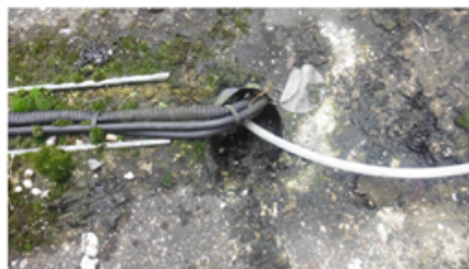
Photo 3 – cabling entering bund floor
