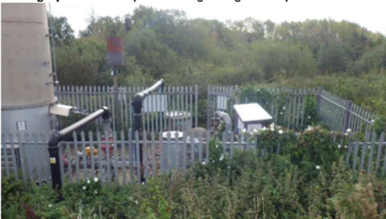
Photograph 2: Gates open for the flare compound.
