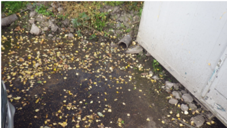
Photograph 6. Pathway for contaminated water to enter ground above canteen on site. Previously raised with operator.
