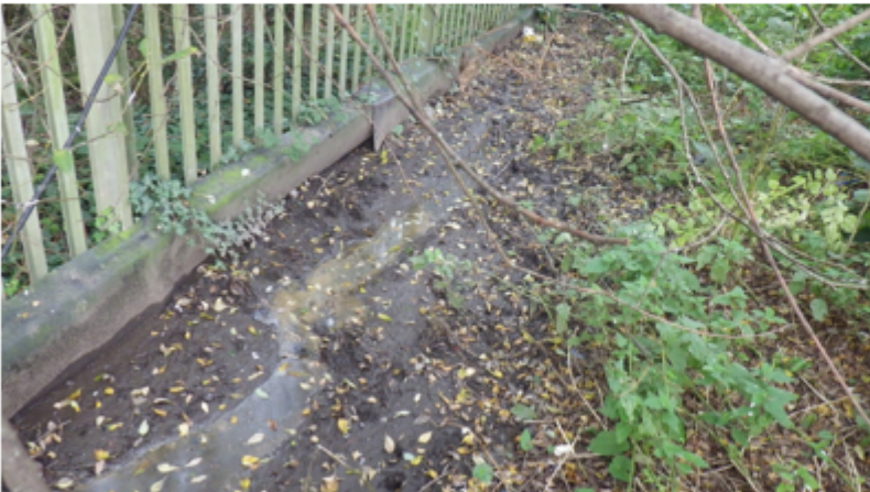
Photograph 5. Evidence of previous emission of contaminated water from the lower transfer station to ground
