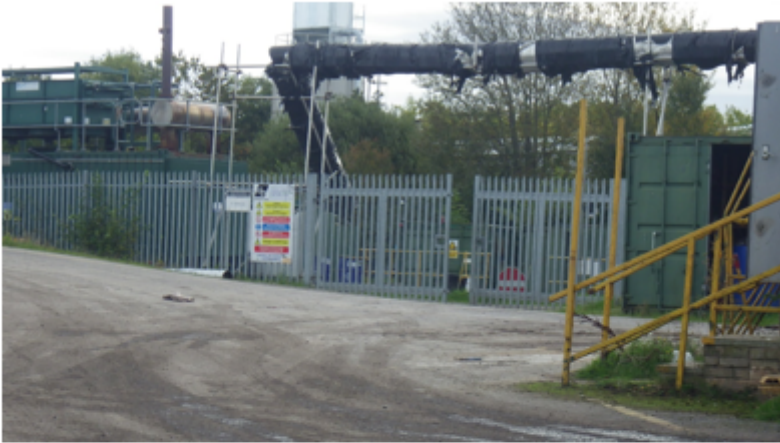
Photograph 1: Gates open for the gas engine compound.
