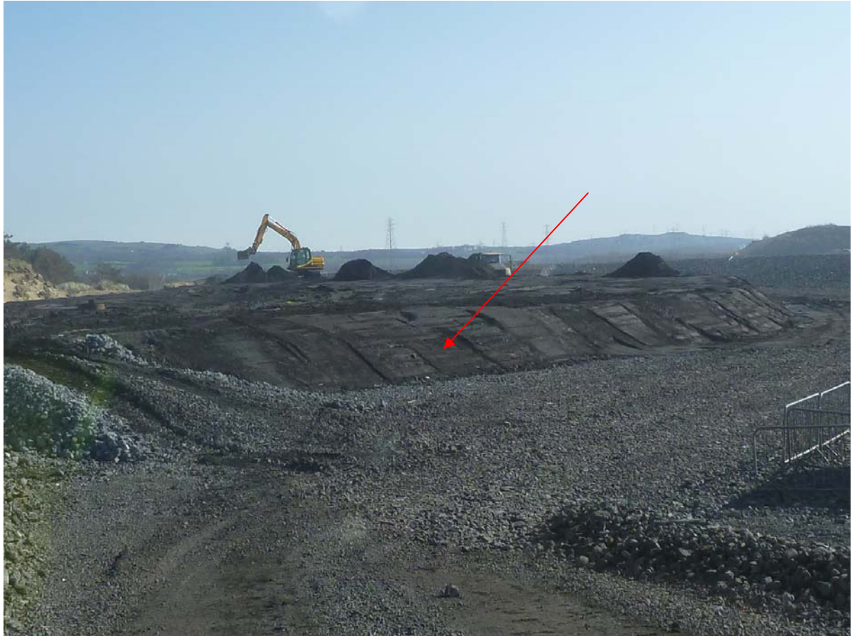
Photograph showing the fire deposit with a thick cover layer (arrow). Hazardous Landfill
