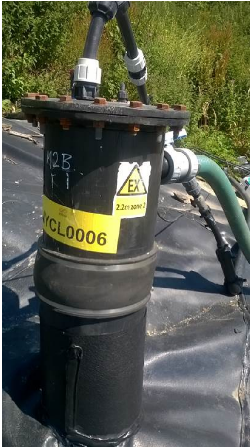
Pic 6. M2B leachate well reacts to the rising leachate level and pumps off the excess to the main holding lagoon. The well pump is powered by an electricity junction box.
