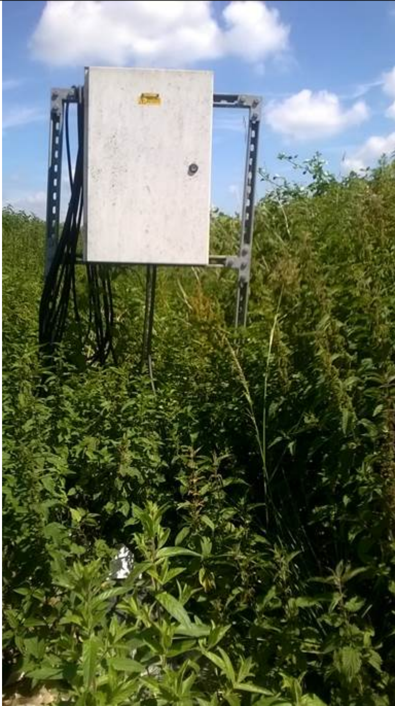
Pic 7. M2B electricity junction box. Site needs to ensure that access remains open to site infrastructure by clearing back the obstructive vegetation.
