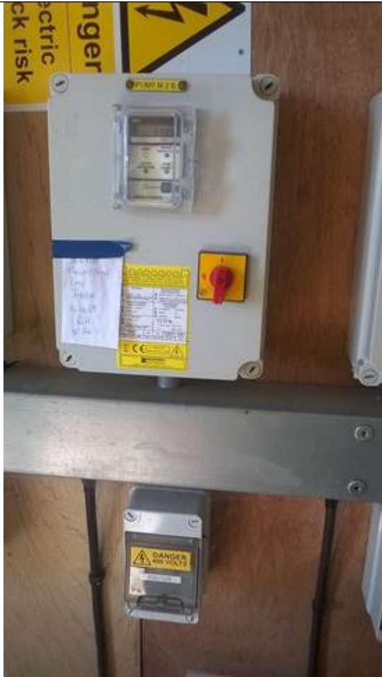
Pic 4. Cell 7 leachate pump control. This is one of 14 similar boxes located between phase 2 and 3. The boxes each log the hour of operation which form the basis of their scheduled maintenance regime. The power supply for the pump control house is via an external generator which is run off diesel which uses approximately 300 litres of diesel per week. Site have previously conducted a feasibility study to run this operation off grid electricity but on balance the generator option is preferred at present.
