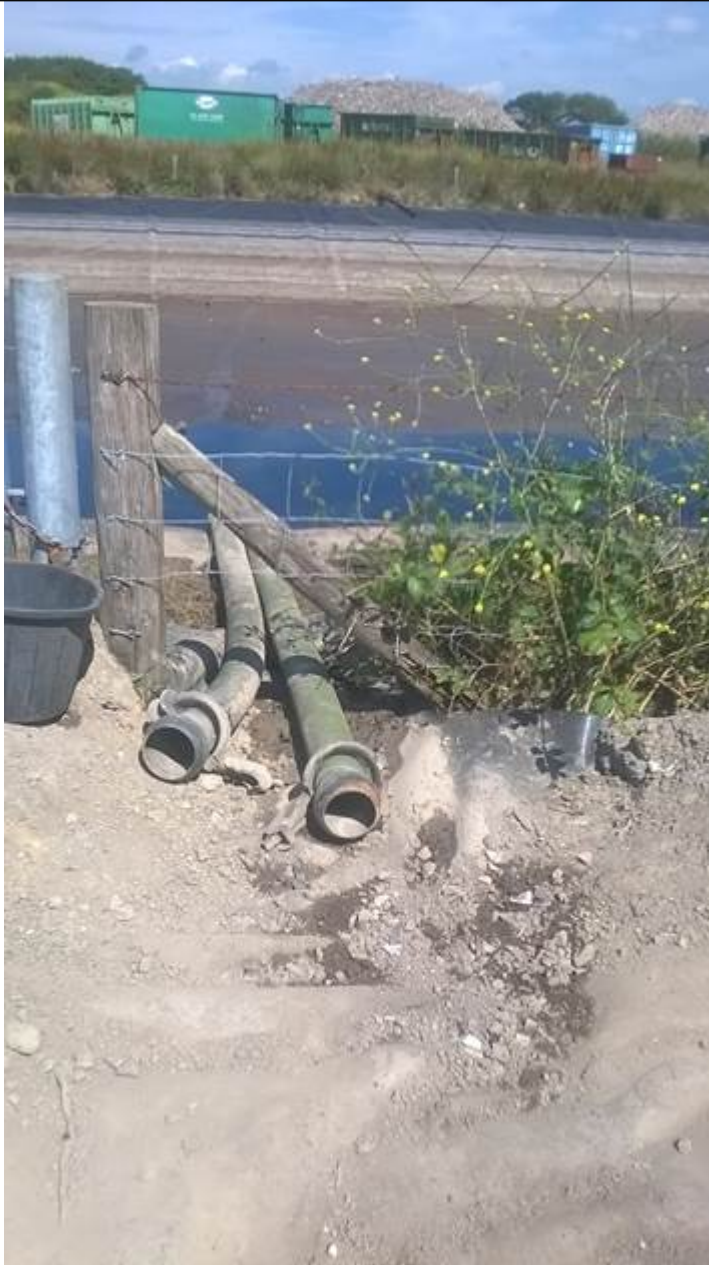
Pic 3. The tanker connection takes place within an engineered bowl which is geotextile lined and flows back to the lagoon. No spillage evidence was seen in this location and the system in place was robust.
