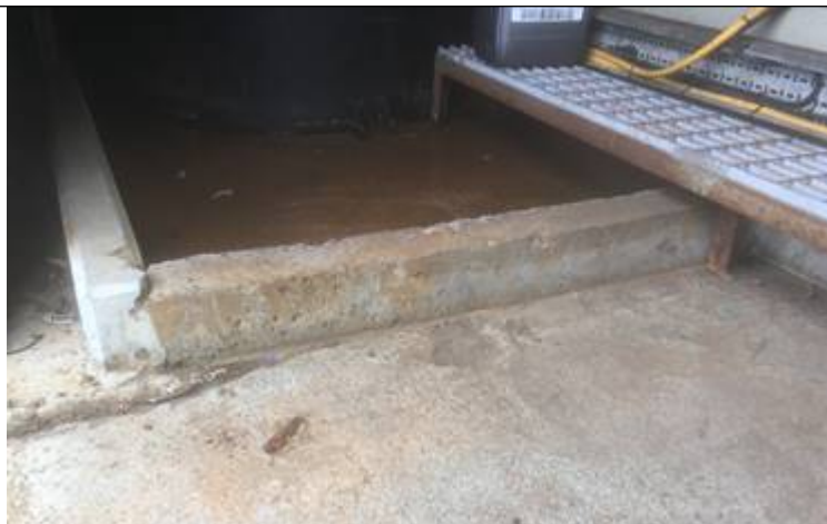
Photo 1 – Deterioration of demin plant bund
