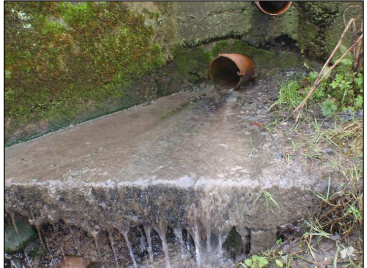
Photo X: Fungus in the vicinity of a discharging surface water drainage outfall.
