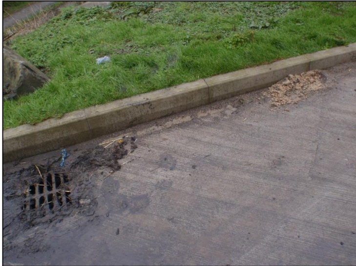
Photo X: raw material spillage near surface water drainage gully as a result of poor house-keeping arrangements.
