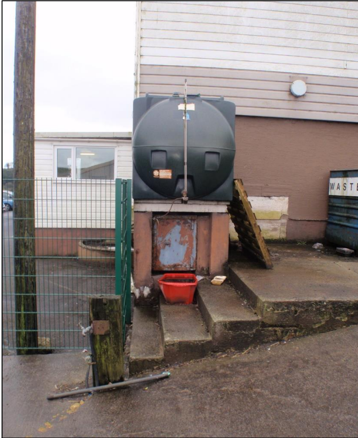
Photo 3: Fuel oil tank adjacent to the main office not served by secondary containment
