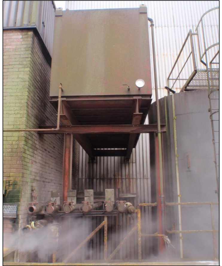
Photo 4: Fuel oil tank adjacent to the site workshop not served by secondary containment.
