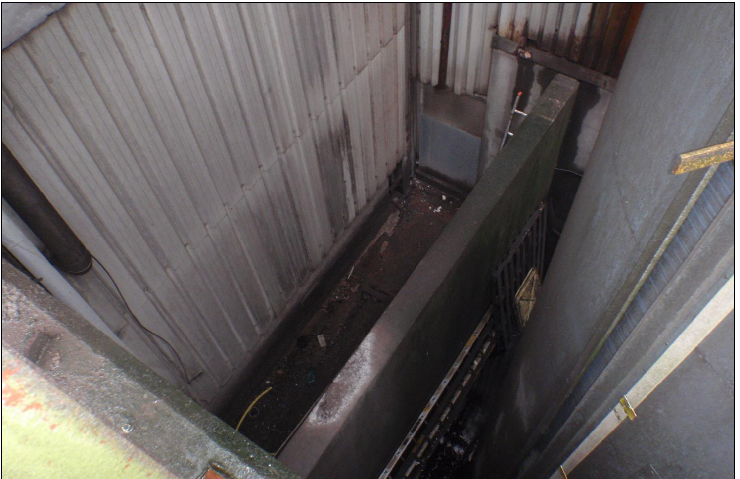
Photo 5: Below the fuel oil tank a partially rendered breeze block partition wall has been constructed. The fuel oil tank is positioned to the left of the partition wall, outside the bunded area. Any leaks (acute or chronic) from the fuel oil tank are therefore not captured by the bund and are able to escape.
