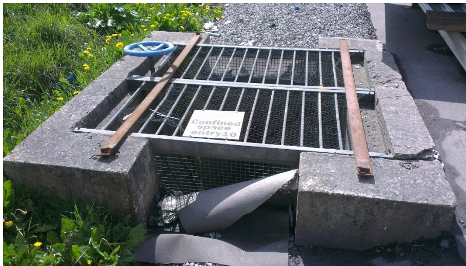
Figures 4: Sealed Infrastructure
