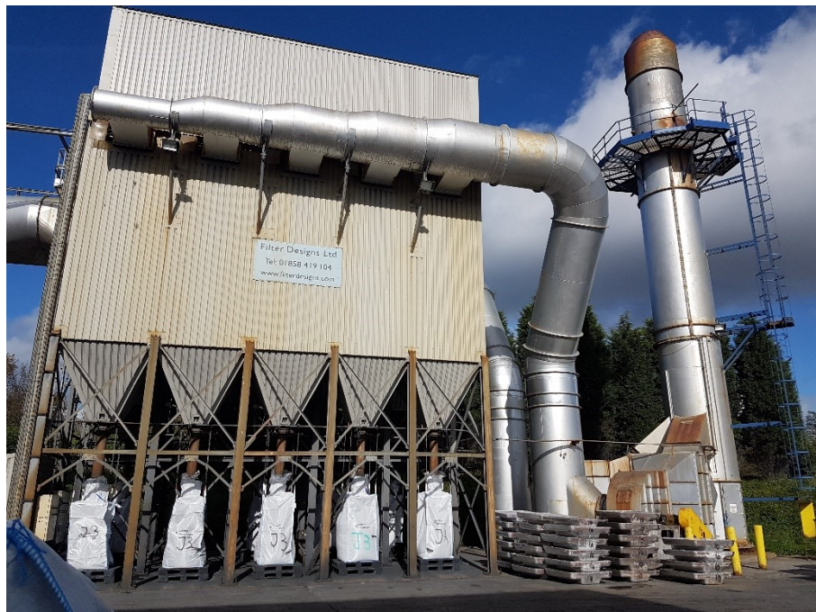
Figure 2: Baghouse and Abatement Extraction
