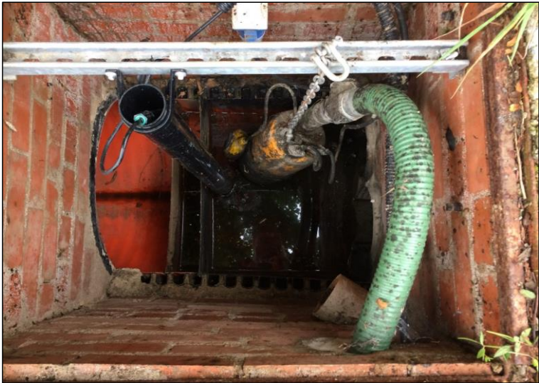
Upstream chamber containing high oil probe and sump pump
