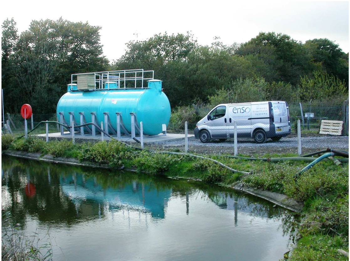
Nant y caws 40 m 3 pilot-scale SAF plant 2011
