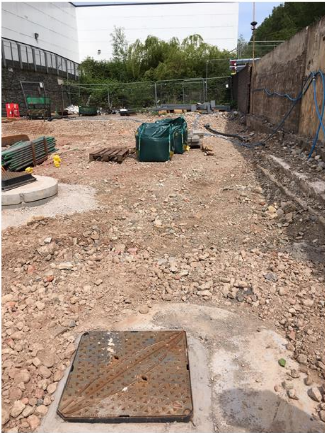
New surface water line carrying Morrisons northern area permitted drainage across 6 th form site
