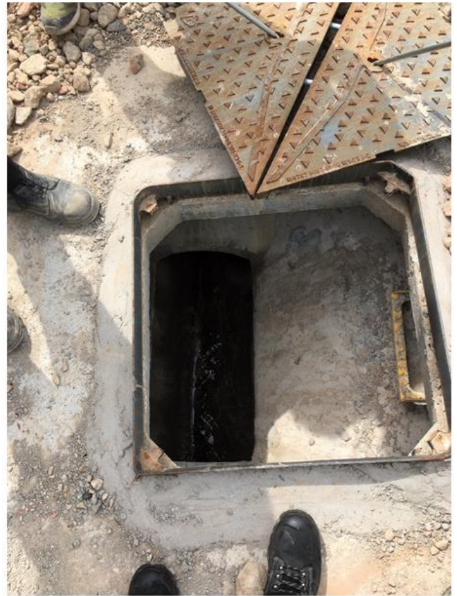
New surface water line manhole lifted. Water flowing despite no rain having fell 1 week before visit
