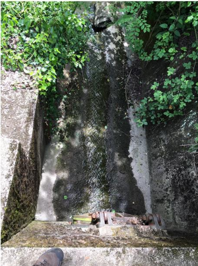
Northern area discharge point into the Afon Lwyd. Discharging despite no rain having fell 1 week before visit
