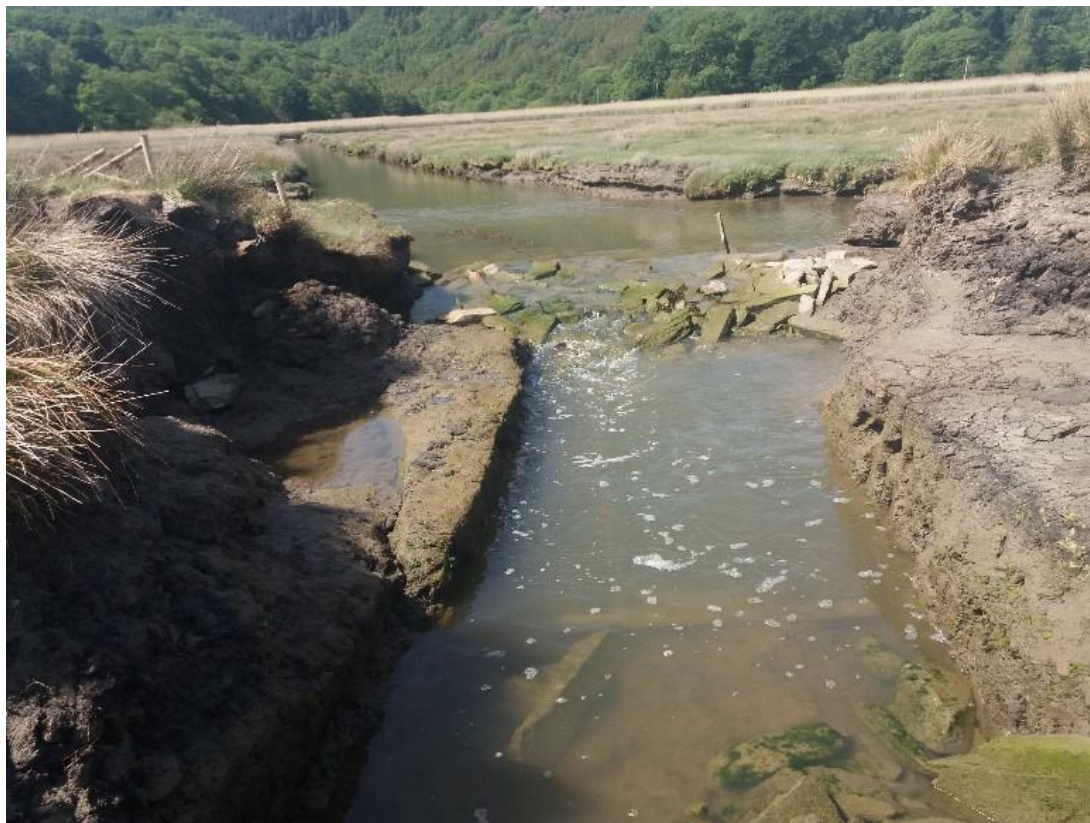
Existing flood bank breach showing extent of vertical scour
