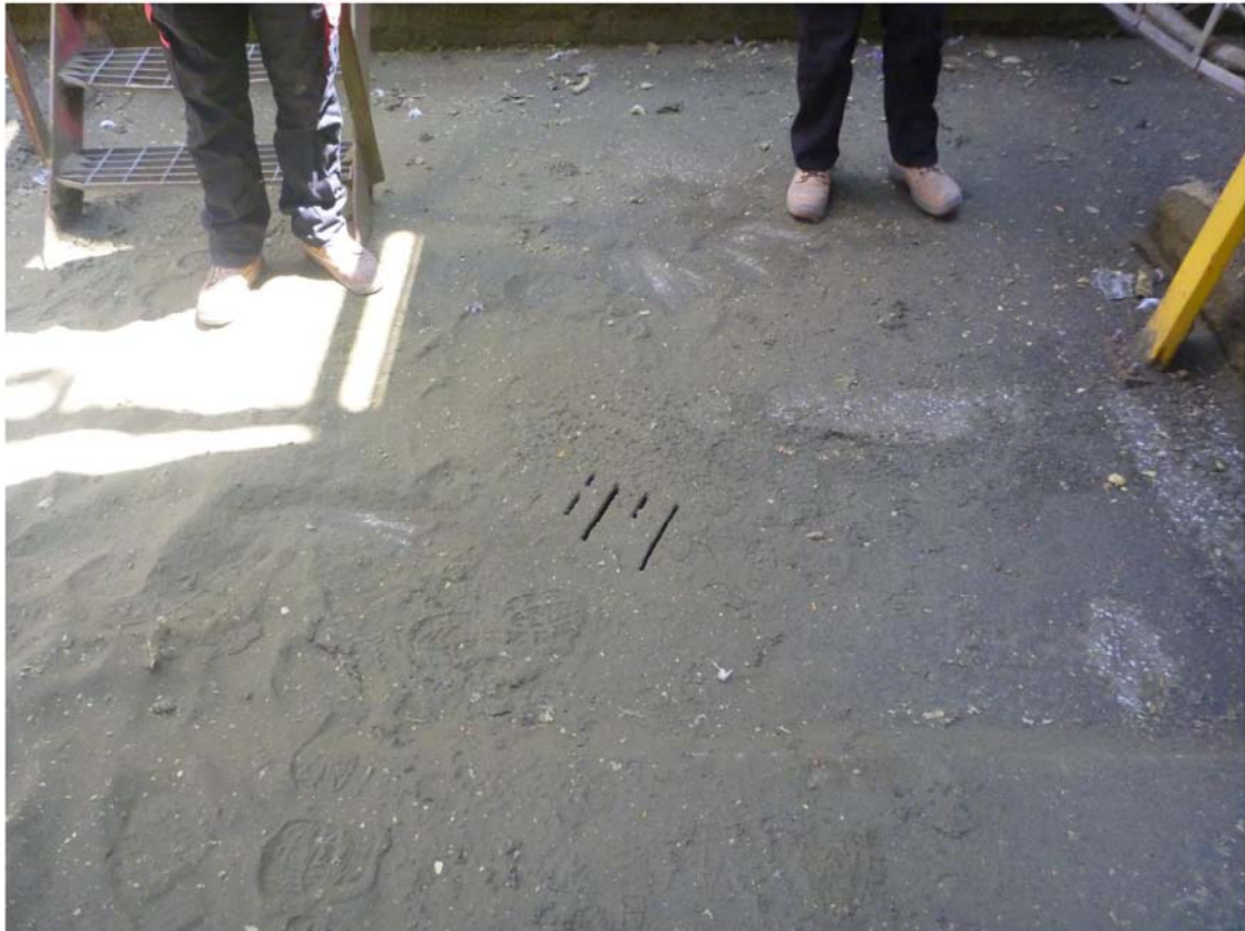
Further dusts/wastes covering drain on yard (adjacent to L1 building)
