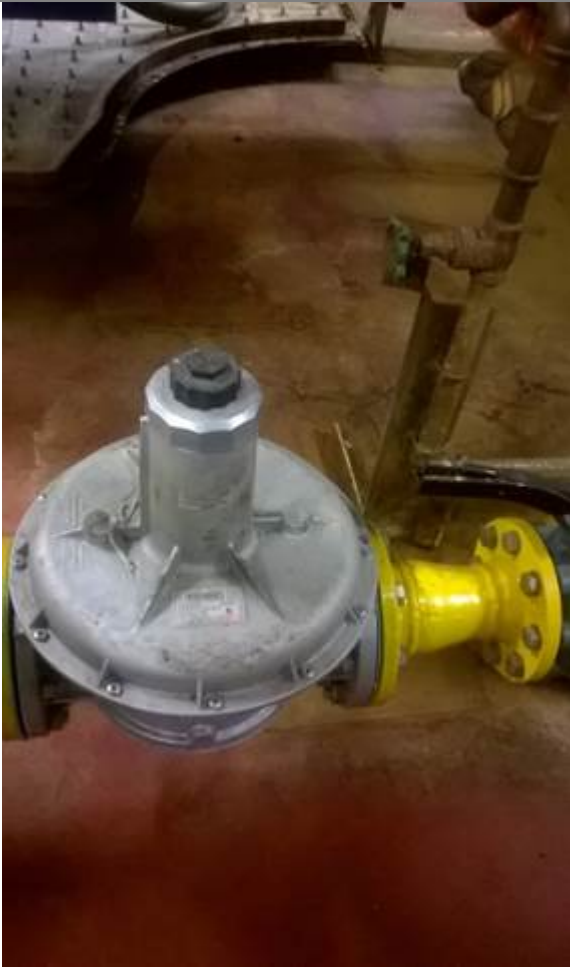
Boiler 4 stage 2 governor is tamper proof sealed.
