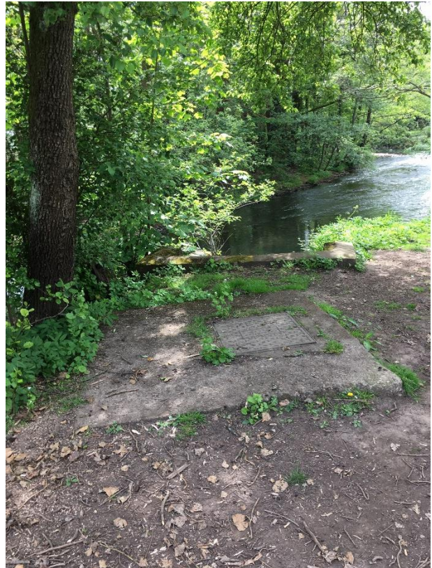
Discharge point and inspection chamber
