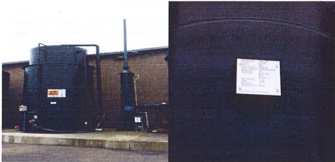
Bulk Nitric Acid Store and scrubber:
