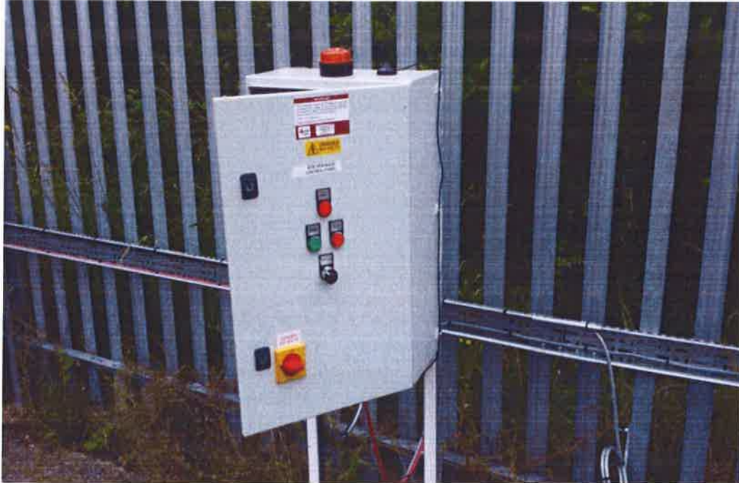
New control panel for SAW pumping system:
