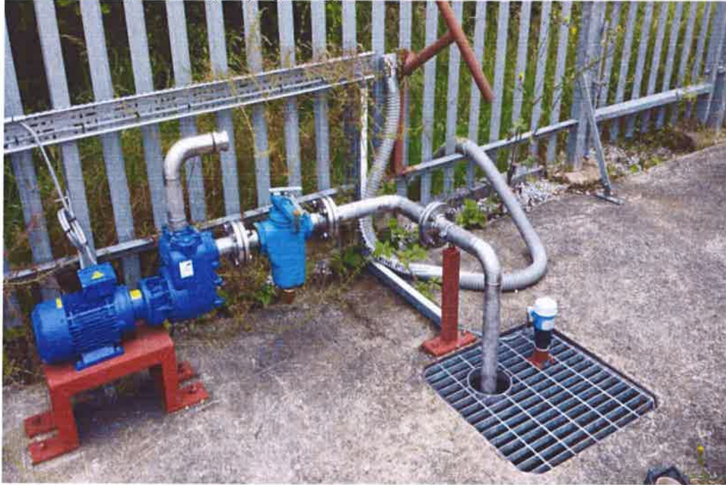
Modified SAW sump with new pumping arrangements:
