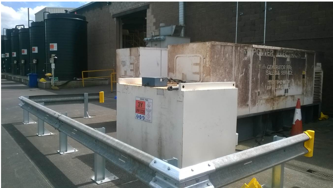
AST Containing Diesel and Power Generator
