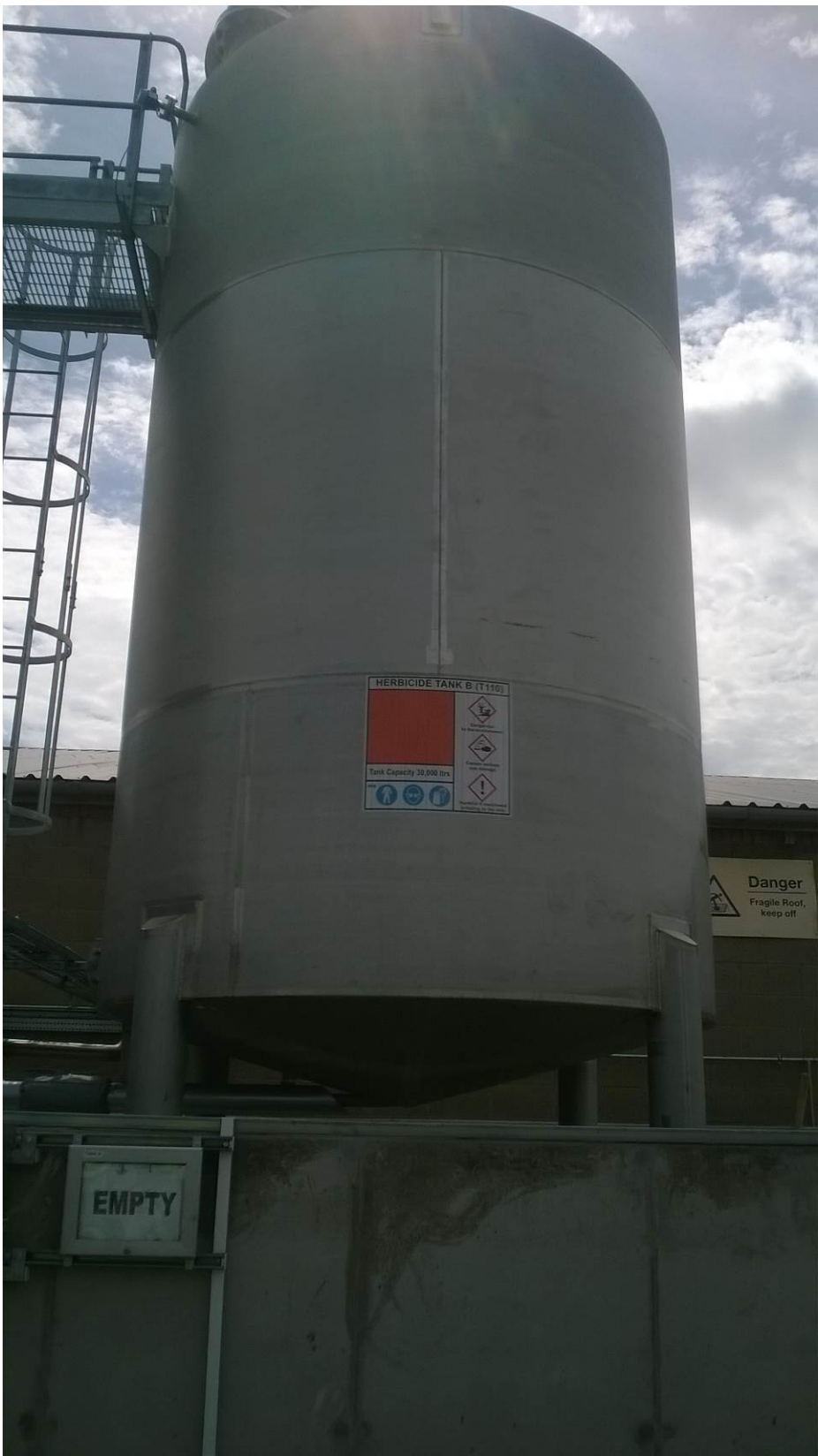
Herbicide Above Ground Storage Tank
