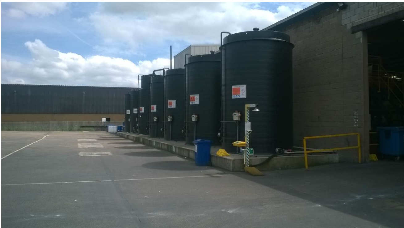
Purpose Built Chemical Storage Tank Farm (ASTs)
