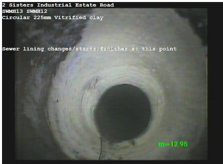
SWMH13X_bacebbe2-a1fc-441e-b5a9-b96c6fbb4217_20170623_154609_181.jpg, 00:01:34, 12.95m Sewer lining changes/starts/finishes at this point
