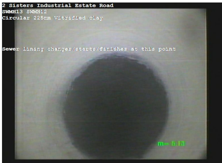
SWMH13X_5f5bbc2f-0c8b-4f0e-badc-9bf328a41d29_20170623_154327_385.jpg, 00:00:16, 5.13m Sewer lining changes/starts/finishes at this point
