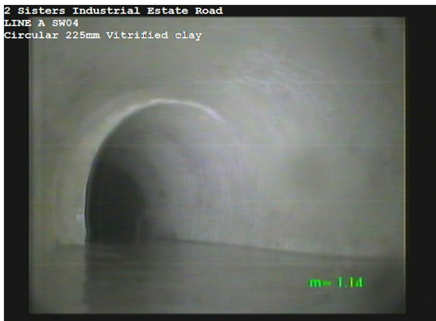
LINE AX_977b7323-0c73-4586-91dc-48bb27dec19d_20170622_160013_701.jpg, 00:00:55, 1.14m Sewer lining changes/starts/finishes at this point
