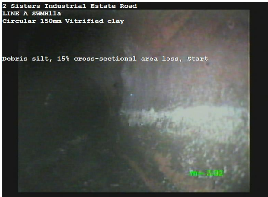
LINE AX_9a7fae94-dcd1-4566-aeb6-42a98a2e9e10_20170622_064255_270.jpg, 00:00:18, 4.19m Debris silt, 15% cross-sectional area loss, Finish
