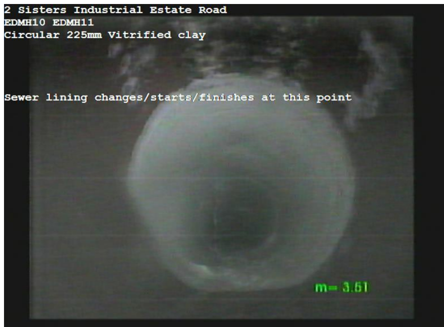
EDMH10X_10becd6d-ca3b-47f4-b675-749b49a00ead_20170623_122402_761.jpg, 00:00:58, 3.51m Sewer lining changes/starts/finishes at this point
