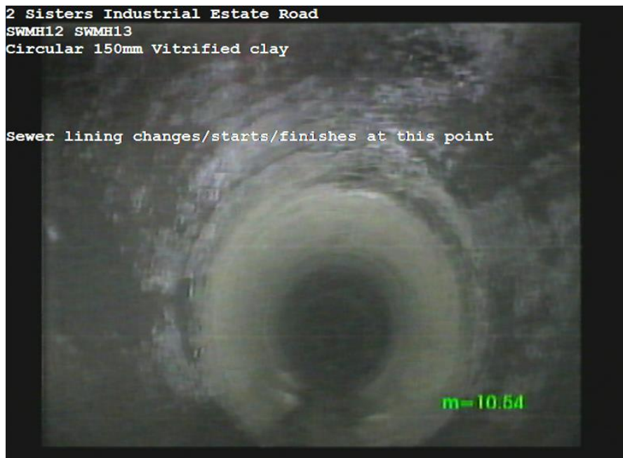
SWMH12X_aec8aa87-c7b4-47b6-9bc8-d217bd1f5245_20170623_160021_820.jpg, 00:00:19, 10.54m Sewer lining changes/starts/finishes at this point
