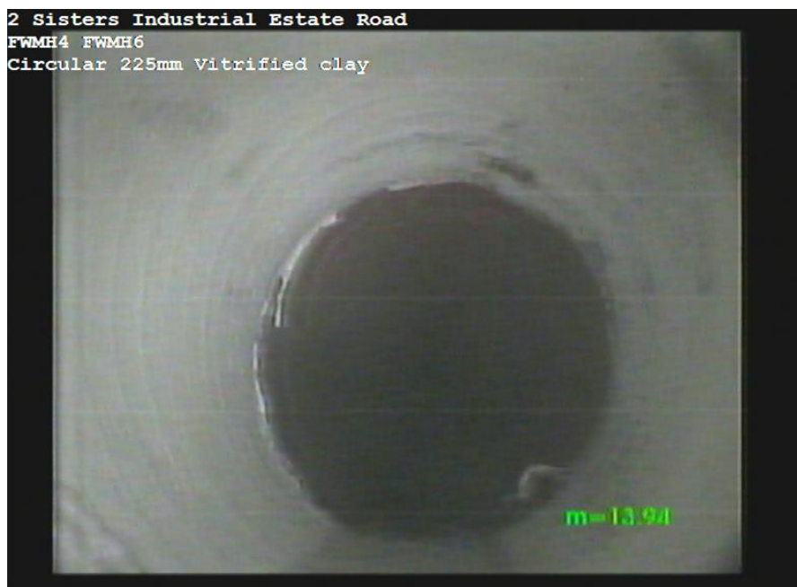
FWMH4X_3f5d34cd-43b8-46bf-a341-98fa62b75929_20170622_124511_205.jpg, 00:02:44, 13.94m Sewer lining changes/starts/finishes at this point
