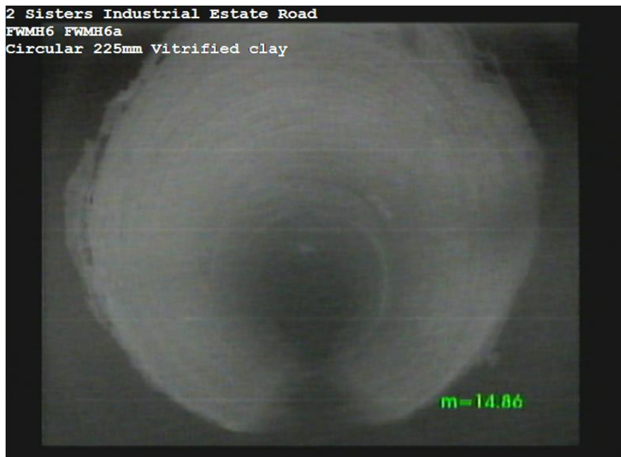
FWMH6X_dfcc0f2a-afa2-4db1-bc94-2e6f148f5554_20170623_161706_052.jpg, 00:02:11, 14.86m Sewer lining changes/starts/finishes at this point
