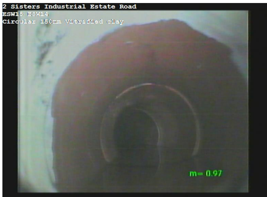
ESW15X_6fe1855c-35e8-4c99-b2ea-e23cb511dbcc_20170623_055102_253.jpg, 00:00:36, 0.97m Sewer lining changes/starts/finishes at this point
