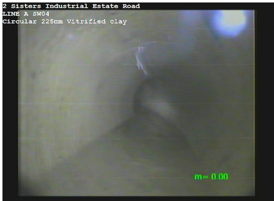
LINE AX_10d967aa-013c-411f-940f-b1f16ea068d3_20170622_155832_243.jpg, 00:00:00, 0.01m Sewer lining changes/starts/finishes at this point
