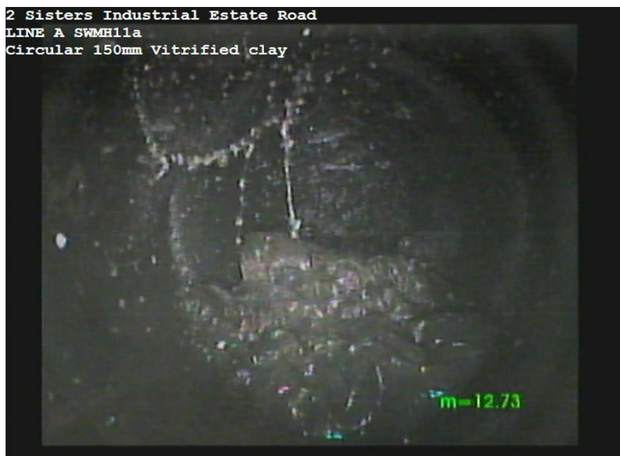
LINE AX_faa065e7-765e-4826-98de-115a3067a3d6_20170622_064632_571.jpg, 00:01:49, 12.73m Obstruction from 12 o'clock to 12 o'clock, 95% height loss
