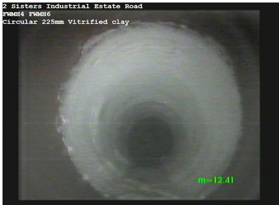
FWMH4X_bd581432-5b32-4c72-bc3b-257f68d926cf_20170622_124544_465.jpg, 00:02:20, 12.44m Sewer lining changes/starts/finishes at this point
