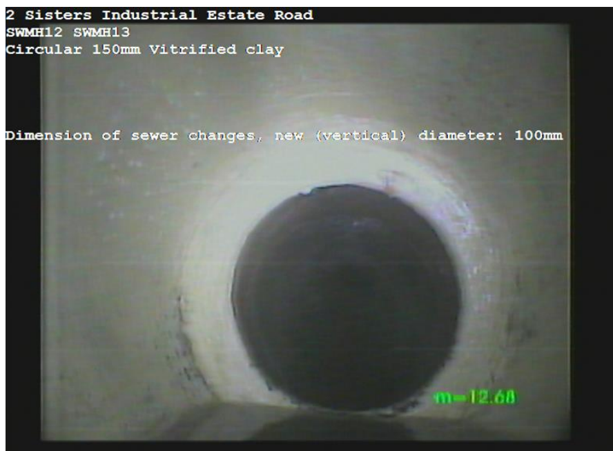
SWMH12X_c8d34e41-a42c-494e-8bee-21741b3b94a9_20170623_160421_393.jpg, 00:02:01, 12.68m Dimension of sewer changes, new (vertical) diameter: 100mm
