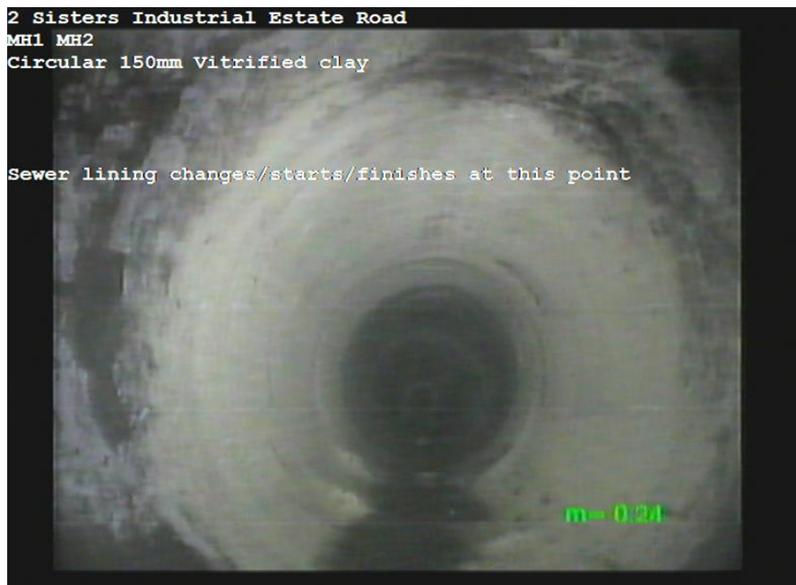
MH1X_1d1fd957-b692-47b7-a99a-d8147e191c6d_20170623_160803_390.jpg, 00:02:11, 0.25m Sewer lining changes/starts/finishes at this point
