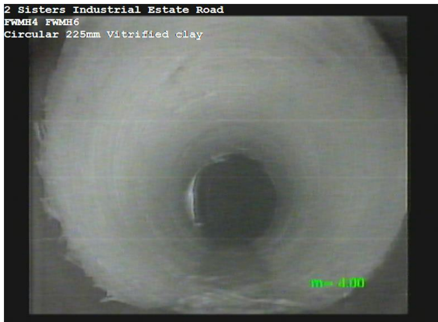
FWMH4X_a5a4e1c0-3f41-46b2-a799-ba14cea9645c_20170622_124154_329.jpg, 00:00:13, 3.92m Sewer lining changes/starts/finishes at this point
