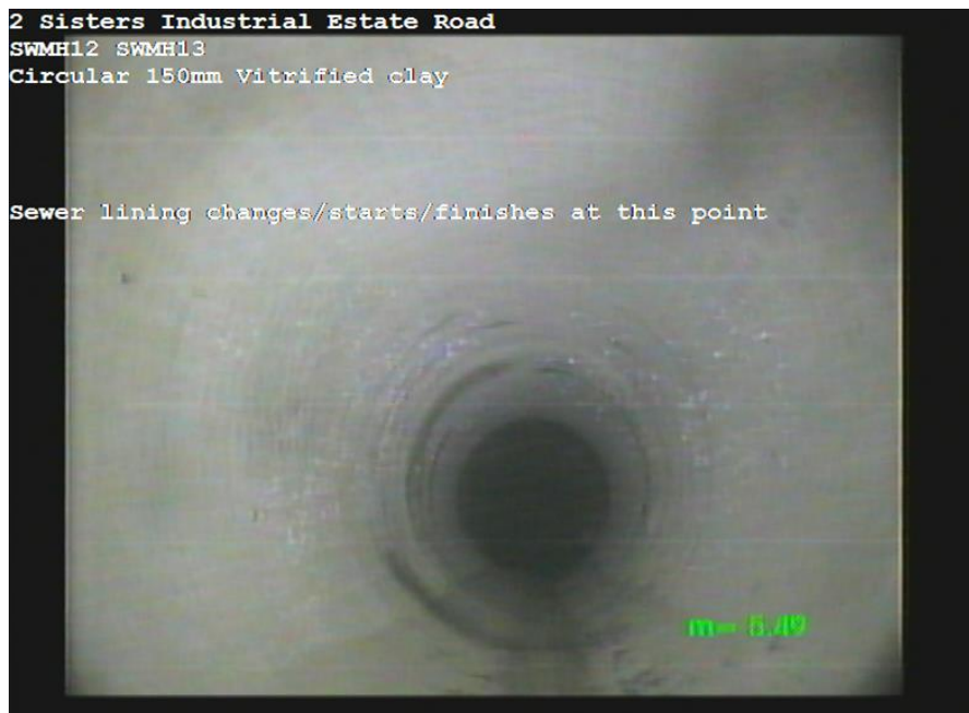
SWMH12X_f37b4eed-09d8-4083-824e-31aa07f8e42c_20170623_155844_389.jpg, 00:02:33, 5.49m Sewer lining changes/starts/finishes at this point
