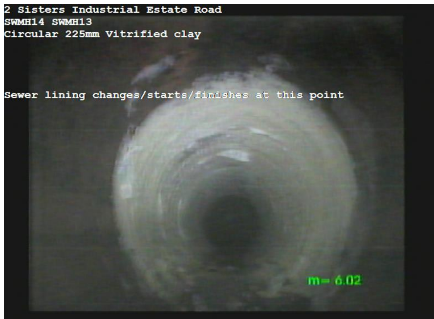
SWMH14X_e0851588-5522-4343-9d17-d992fabaab4a_20170623_153331_869.jpg, 00:02:19, 5.94m Sewer lining changes/starts/finishes at this point
