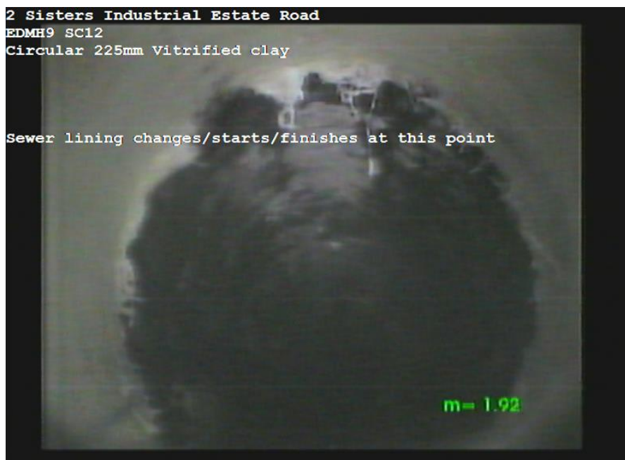
EDMH9X_1c9921d1-9b57-4d02-b12d-2d46032187ea_20170623_115512_696.jpg, 00:00:35, 1.92m Sewer lining changes/starts/finishes at this point
