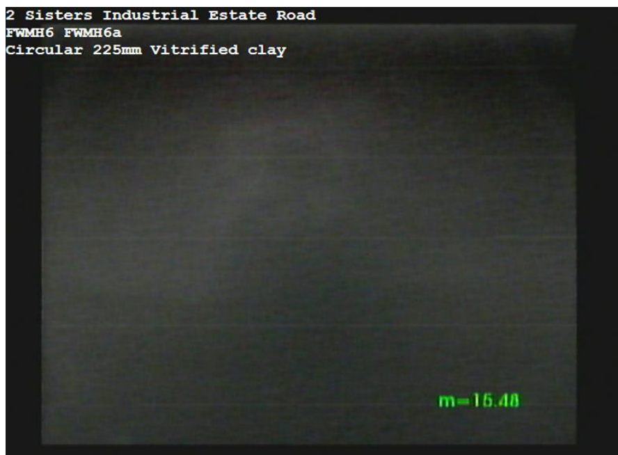
FWMH6X_daff379e-f0fc-4b2e-9292-191b6c348b9d_20170623_161818_438.jpg, 00:02:11, 15.48m Sewer lining changes/starts/finishes at this point
