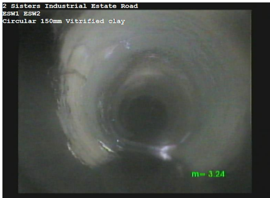
ESW1X_4b29e6cd-490b-47bc-83e7-2f95f5e0d252_20170623_060337_733.jpg, 00:00:22, 3.24m Sewer lining changes/starts/finishes at this point
