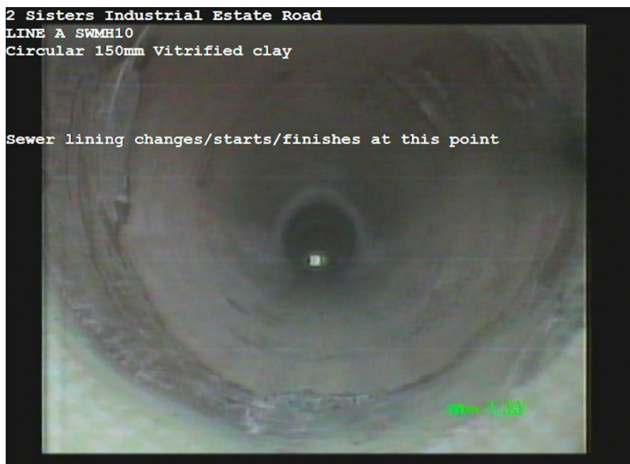
LINE AX_84deb483-3fef-402f-b2ed-e27d9877b0ef_20170620_114232_648.jpg, 00:00:34, 1.33m Sewer lining changes/starts/finishes at this point
