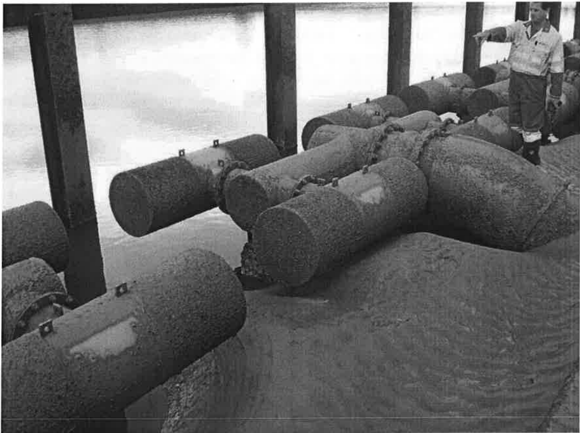
Figure 1. PWWC screening at Connahs Quay. Significant biofilm accumulation is clearly visible on the mesh screens.
