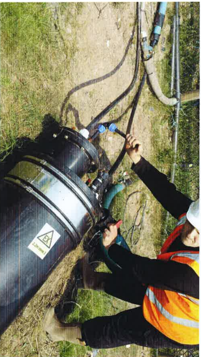
5. Leachate side riser 2. 8000ppm at head of riser, possibly due to redundant leaking pneumatic pump exhaust.
