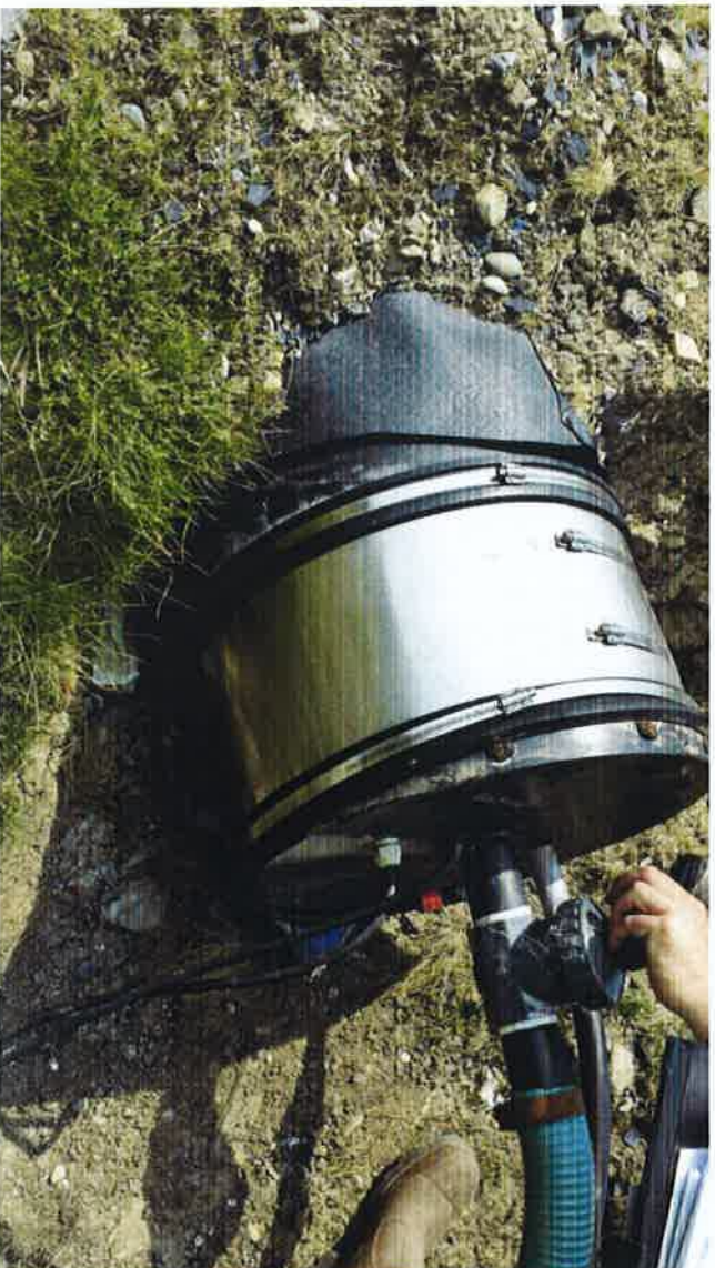
4. Leachate Side Riser 1 – Odour noted downwind of well and elevated methane emissions noted from boot detail.
