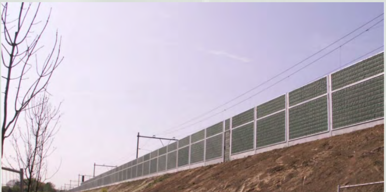
CANOR BENELUX BV noisebarriers
