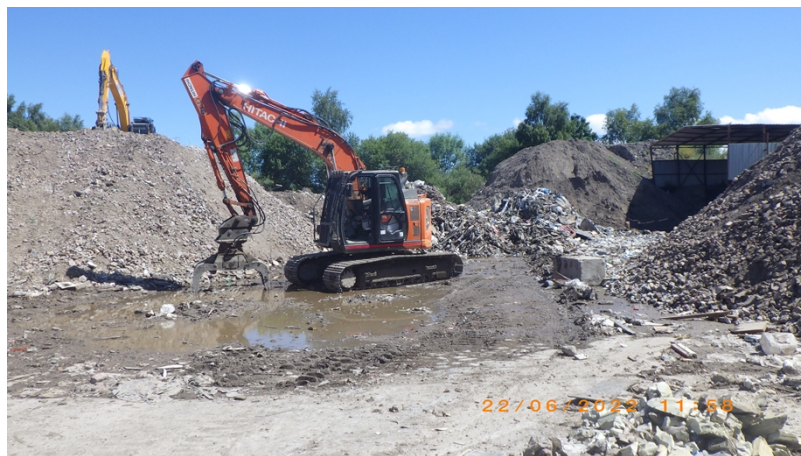
Fire damaged waste to rear of digger
