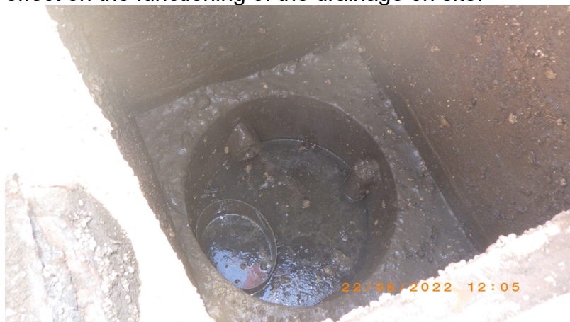
Interceptor on site
