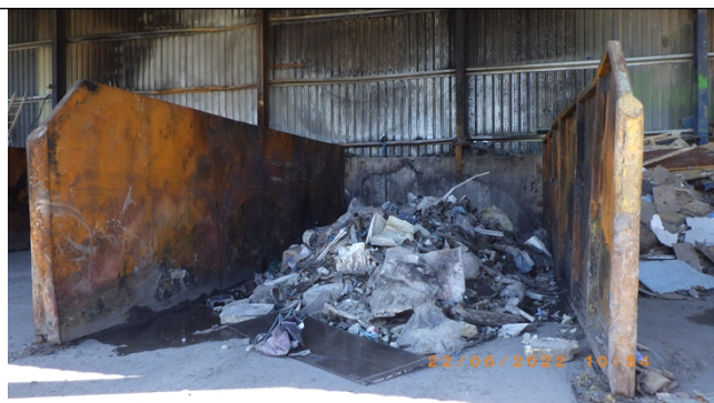
Fire damage on site
