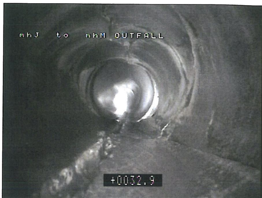
Photo: 96_23a, Tape No.: 01, 00:04:46 33m, Circumferential Fracture, from 12 to 05 o'clock
