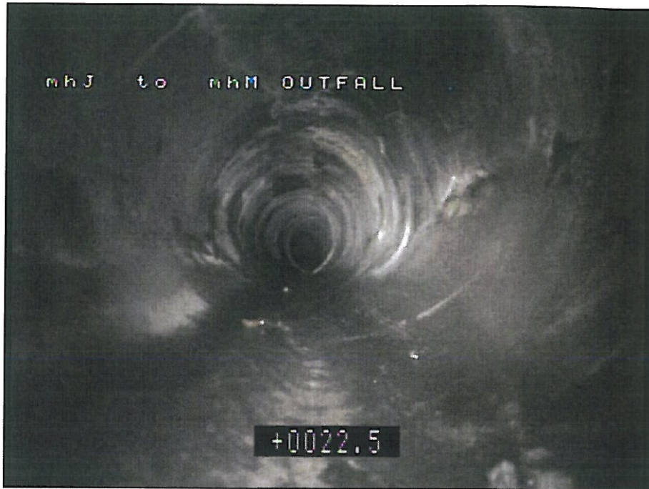
Photo: 9_11b, Tape No.: 01, 00:03:12 22.4m, Connection defective, at 02 o'clock, dia 100 mm
