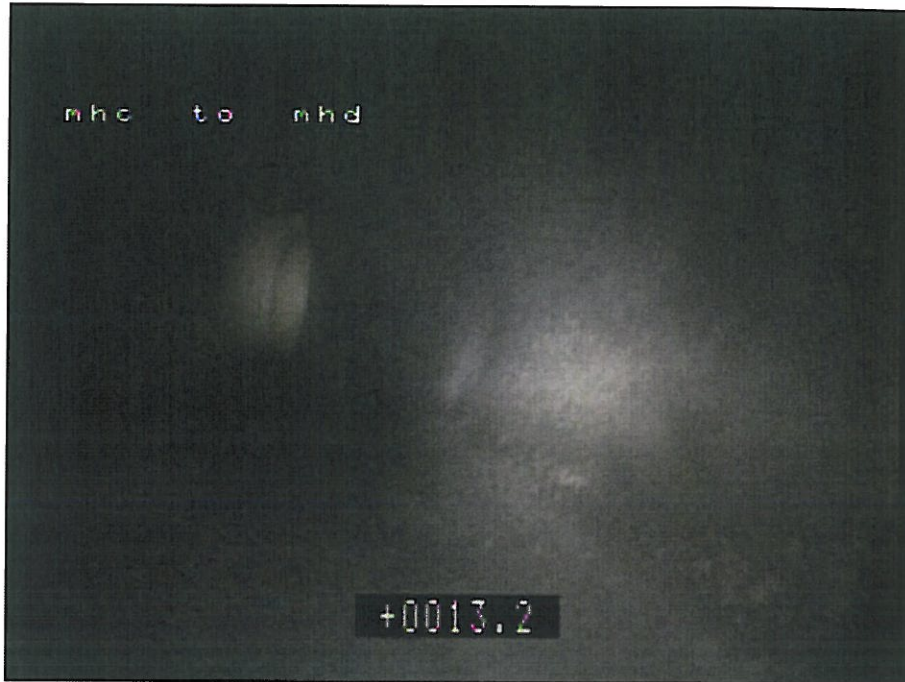
Photo: 36_4a, Tape No.: 01, 00:02:07 13.9m, Connection defective, at 09 o'clock, dia 100 mm, intrusion 50 mm
