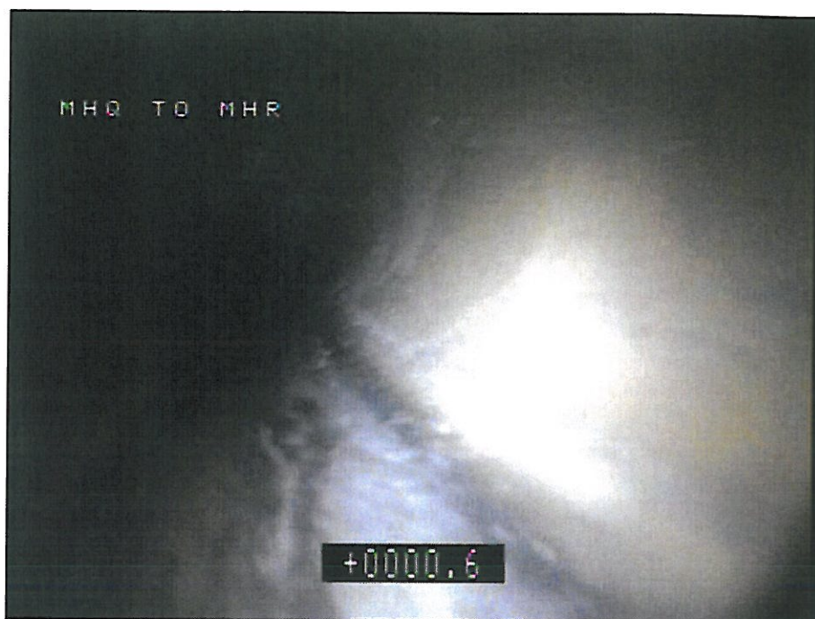
Photo: 113_3a, Tape No.: 01, 00:00:00 0m, Water level, 05 % height/diameter
