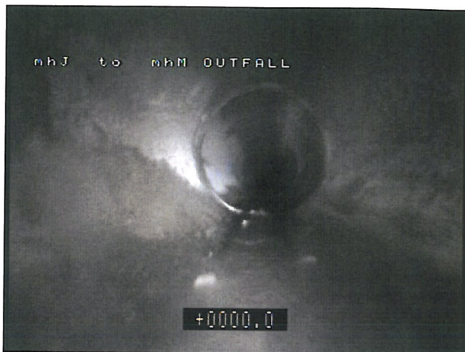
Photo: 74_3a, Tape No.: 01, 00:00:00 0m, Water level, 05 % height/diameter
