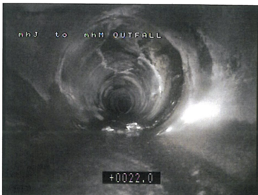
Photo: 9_11a, Tape No.: 01, 00:03:12 22.4m, Connection defective, at 02 o'clock, dia 100 mm
