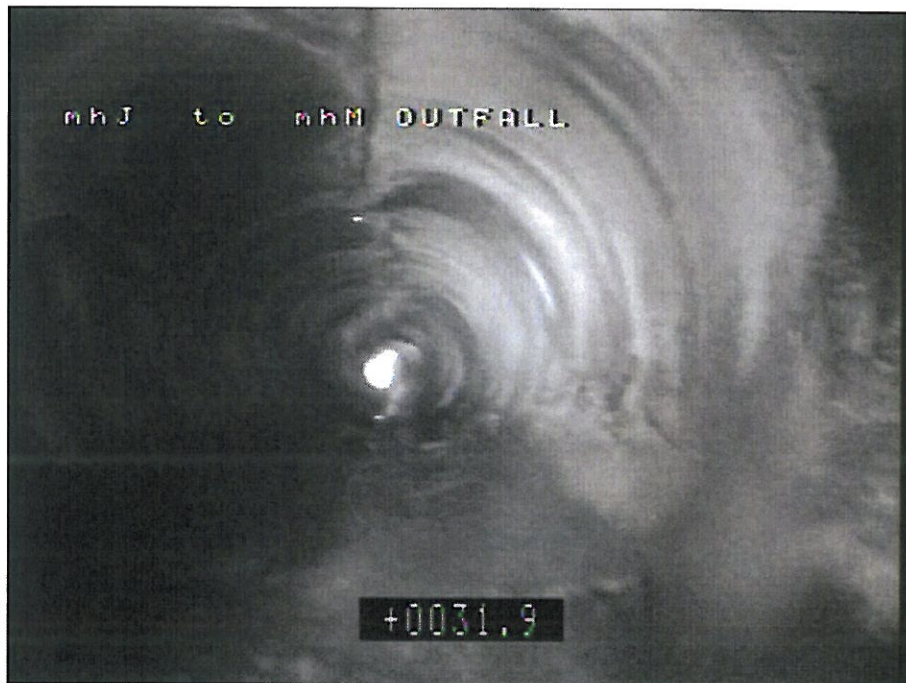
Photo: 9_20a, Tape No.: 01, 00:04:22 31.9m, Sewer Deformed, 10 %
