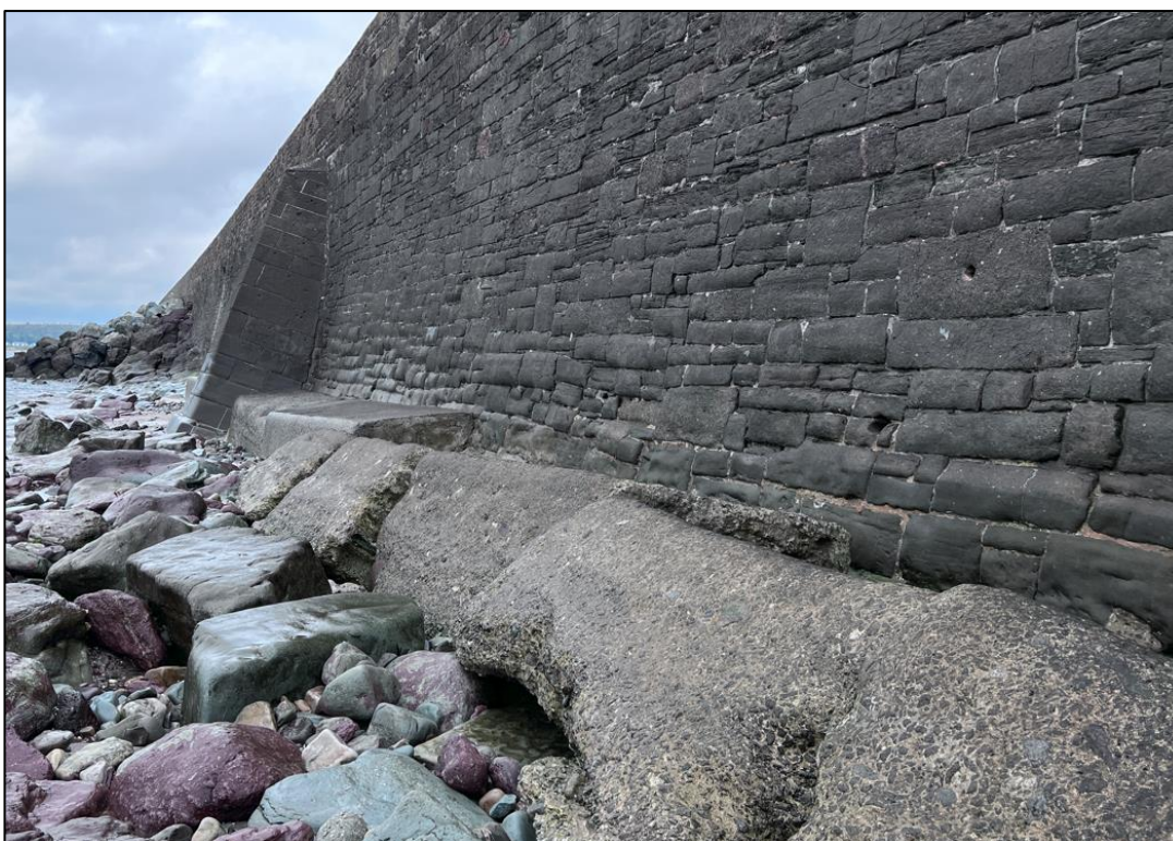
Figure 2: Toe bean failure below Saint Ishmaels Sea Defence
