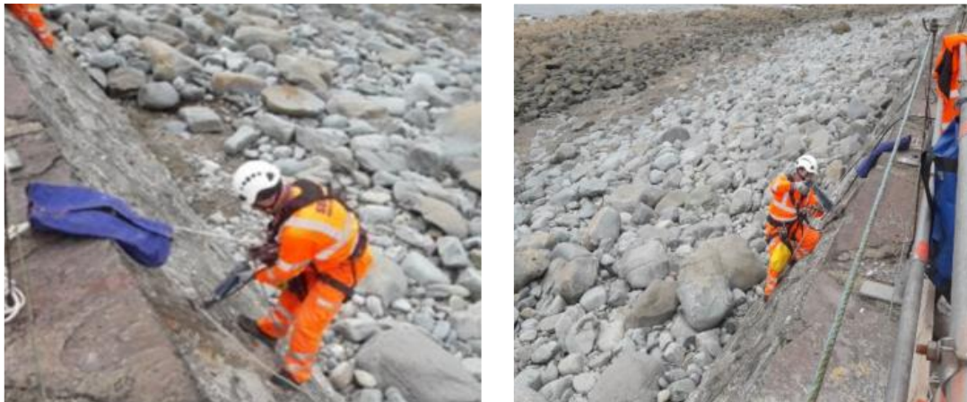
Figure 4: Selection of images of previous minor wall repairs on a different rail route.
