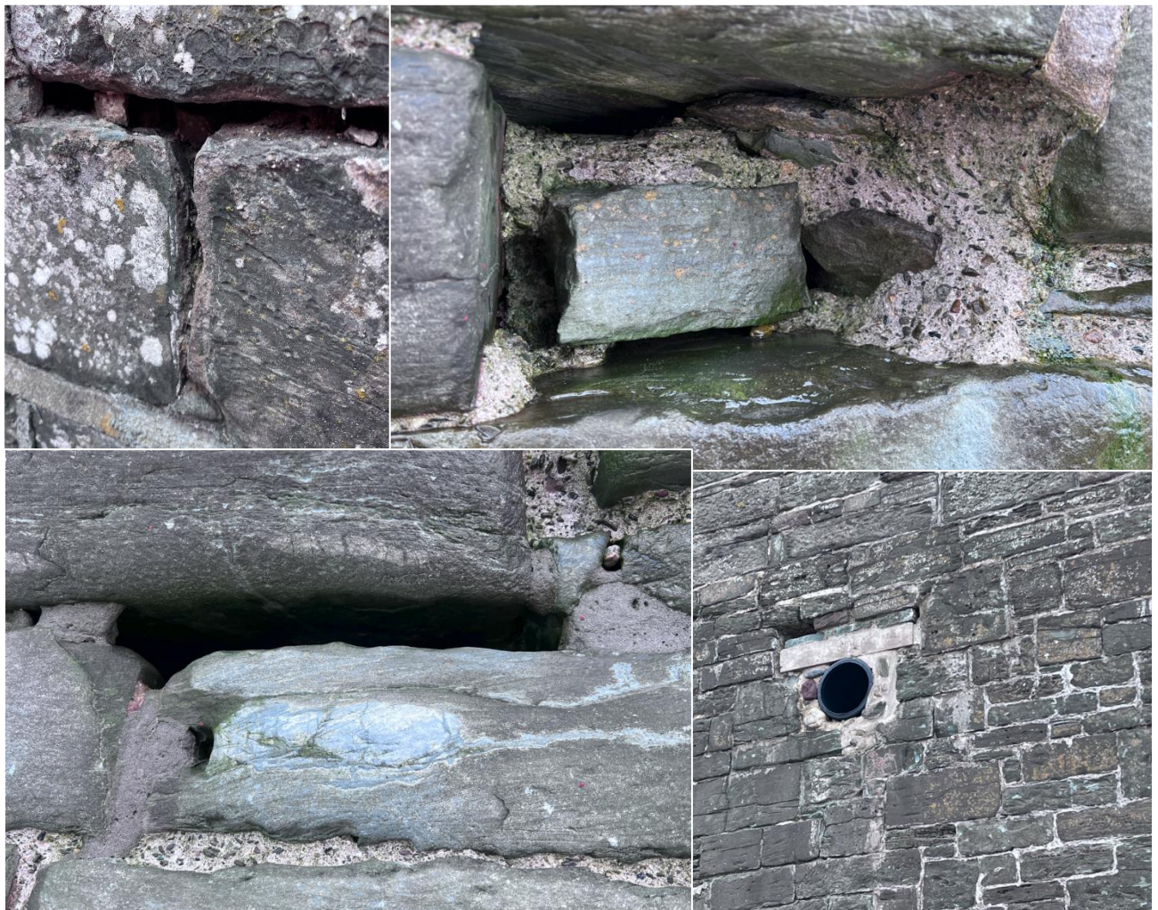
Figure 5: The figure above provides a visual assessment wall during 2022.
