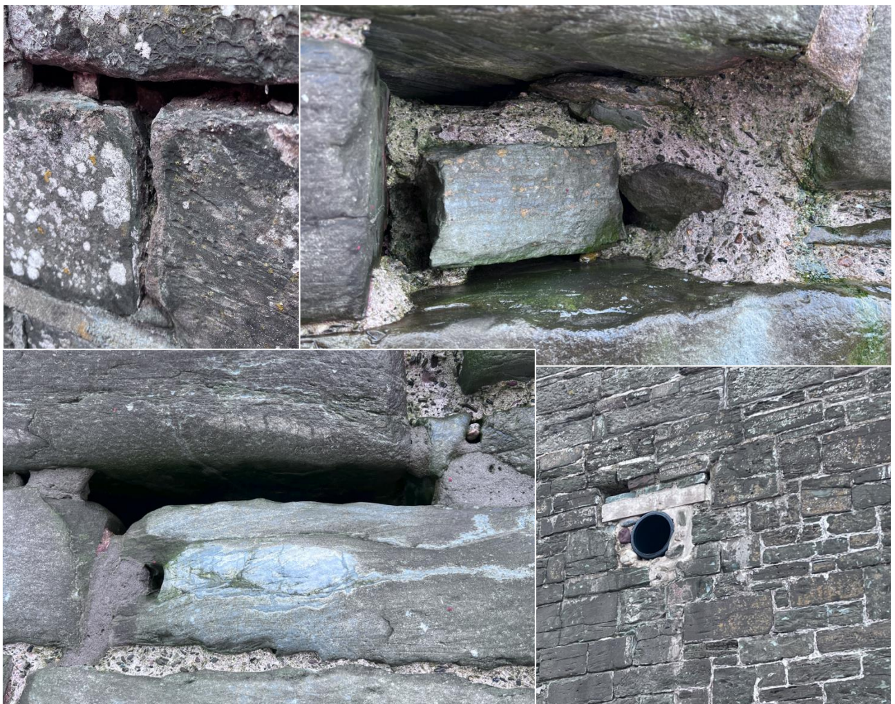
Figure 3: The figure above provides a visual assessment of the 2020 condition of some SWM2 Sea Wall observed using a drone recording camera, (Images from spring 2020, via Network Rail).
