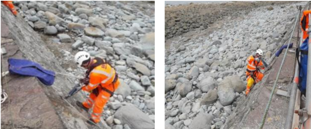
Figure 2: Selection of images of previous minor wall repairs on a different rail route.
