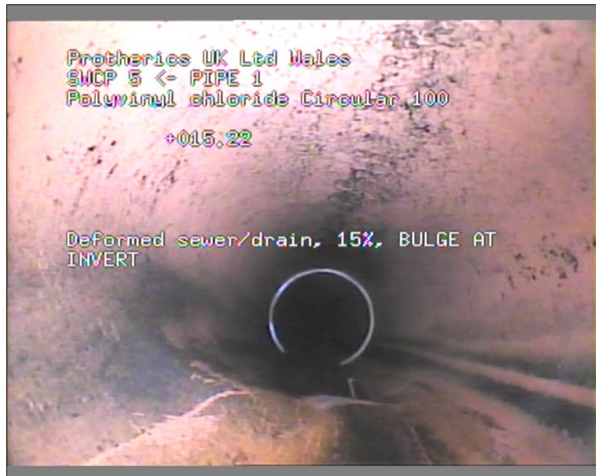
Photo: 39_39_246_A.JPG 15.22m, Deformed sewer/drain, 15%
