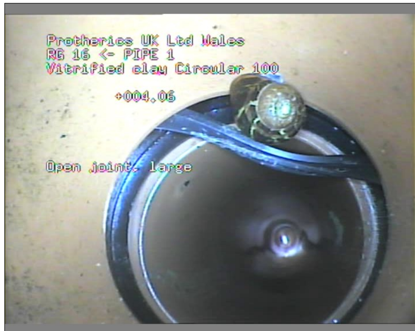
Photo: 32_32_192_A.JPG 4.06m, Open joint, large
