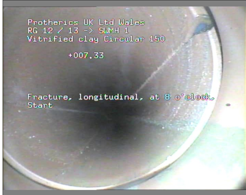
Photo: 18_18_102_A.JPG 7.33m, Fracture, longitudinal, at 8 o'clock, Start
