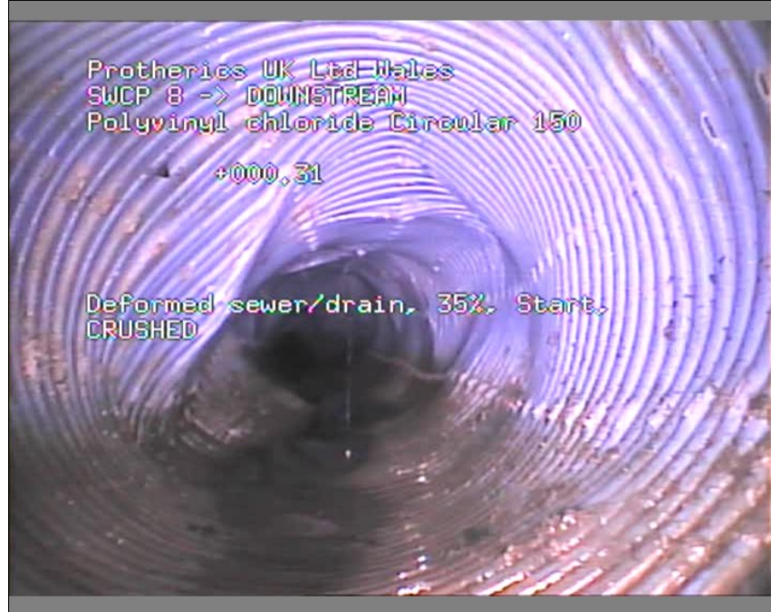
Photo: 47_47_288_A.JPG 0.31m, Deformed sewer/drain, 35%, Start
