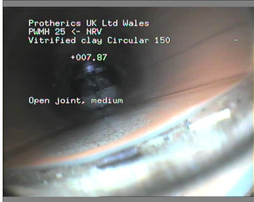
Photo: 126_126_832_A.JPG 7.87m, Open joint, medium
