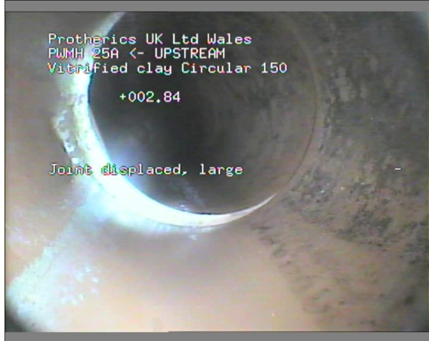
Photo: 131_131_865_A.JPG 2.84m, Joint displaced, large
