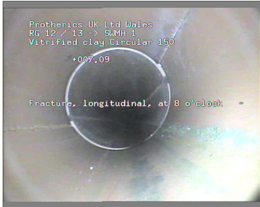
Photo: 18_18_100_A.JPG 7.09m, Fracture, longitudinal, at 8 o'clock
