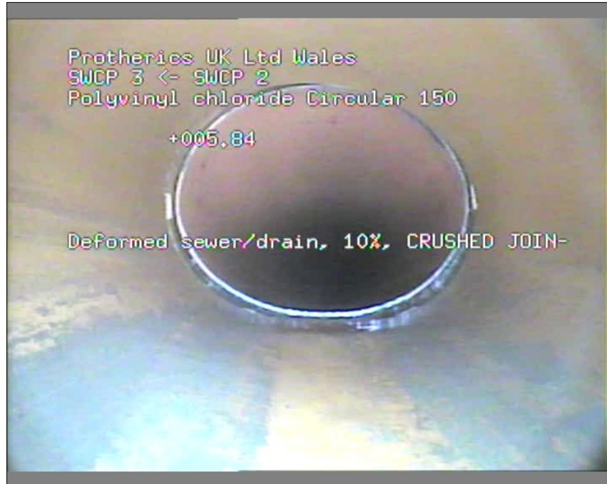
Photo: 27_27_161_A.JPG 5.84m, Deformed sewer/drain, 10%
