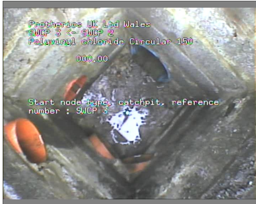
Photo: 27_27_155_A.JPG 0m, Start node type, catchpit, reference number : SWCP 3
