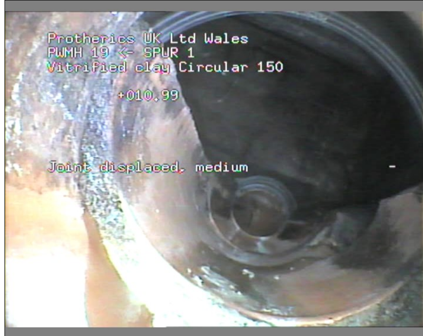
Photo: 113_113_733_A.JPG 10.99m, Joint displaced, medium
