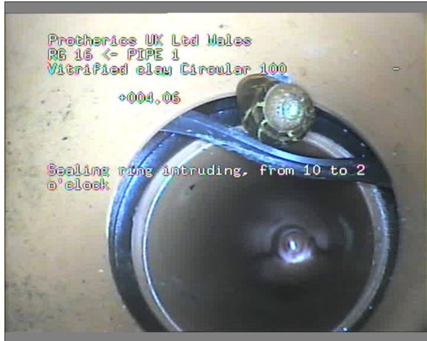
Photo: 32_32_193_A.JPG 4.06m, Sealing ring intruding, from 10 to 2 o'clock
