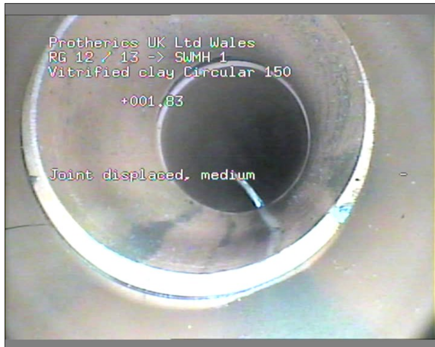
Photo: 18_18_95_A.JPG 1.83m, Joint displaced, medium
