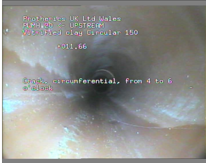
Photo: 115_115_753_A.JPG 11.66m, Crack, circumferential, from 4 to 6 o'clock
