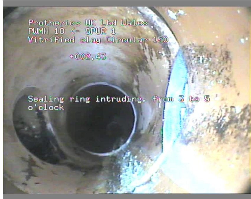
Photo: 111_111_712_A.JPG 2.43m, Sealing ring intruding, from 3 to 5 o'clock
