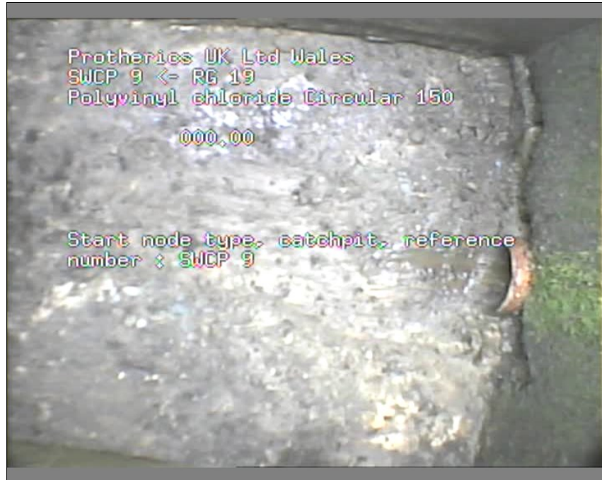
Photo: 50_50_312_A.JPG 0m, Start node type, catchpit, reference number : SWCP 9
