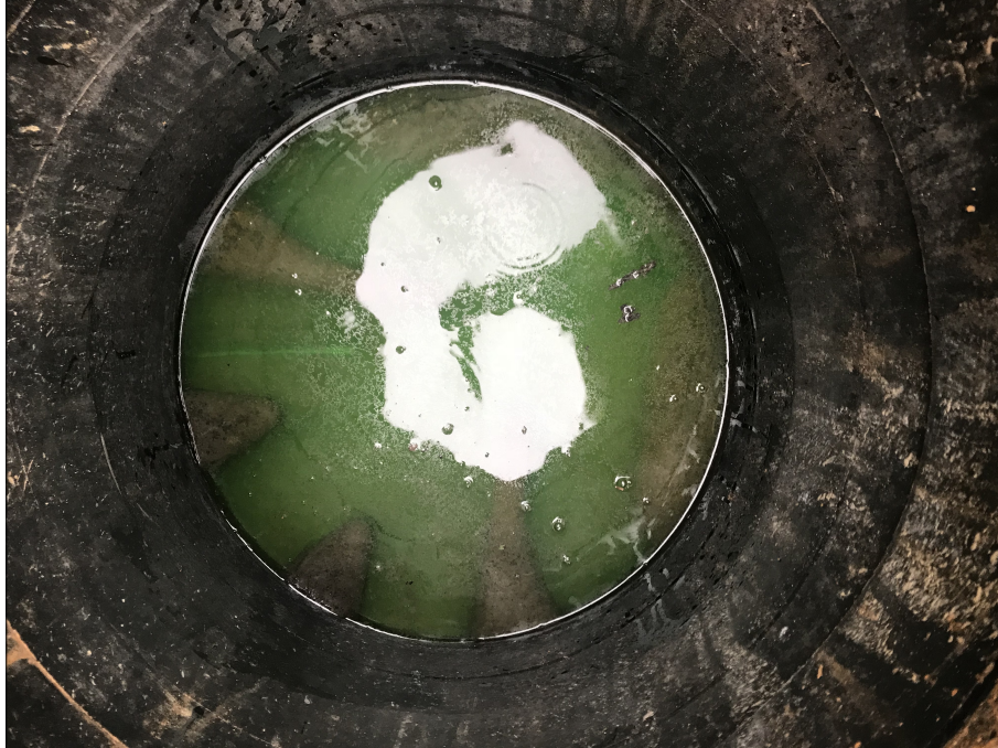
Photo: FWMH 1 Surcharged.JPG 0m, General remark
