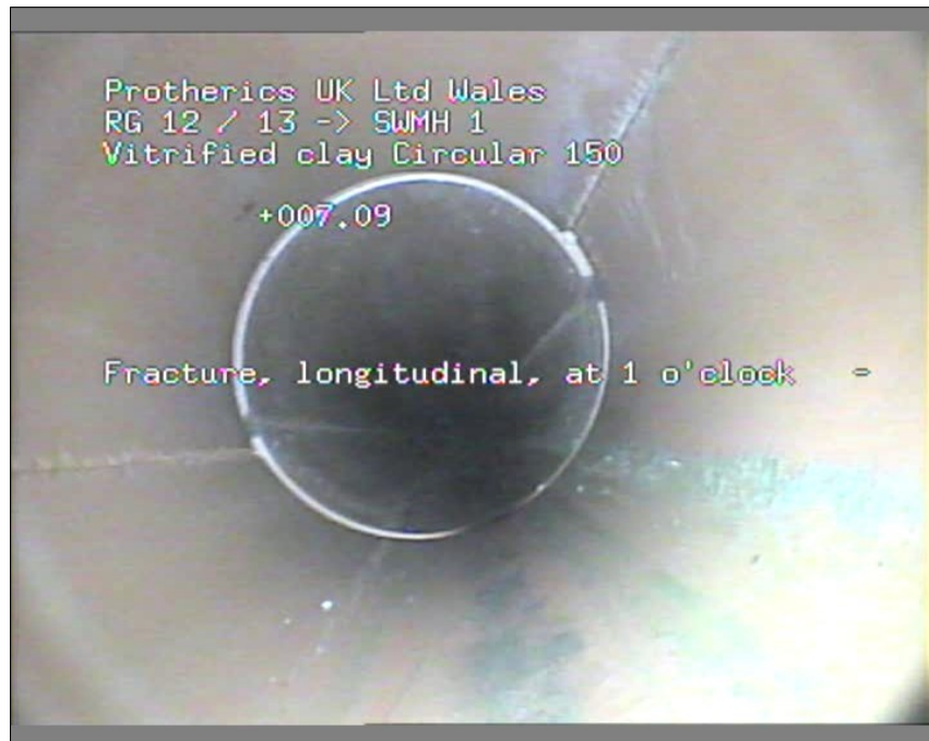
Photo: 18_18_99_A.JPG 7.09m, Fracture, longitudinal, at 1 o'clock
