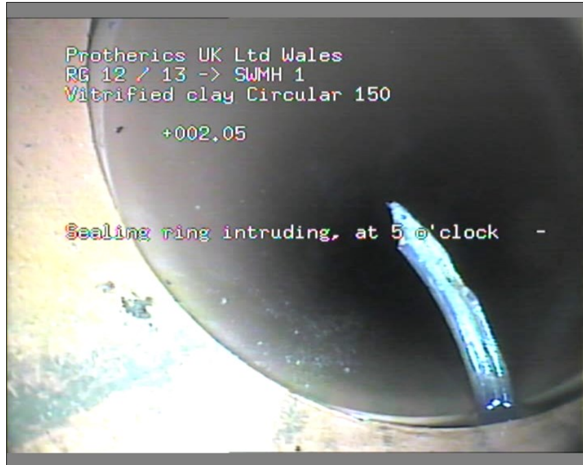
Photo: 18_18_97_A.JPG 2.05m, Sealing ring intruding, at 5 o'clock
