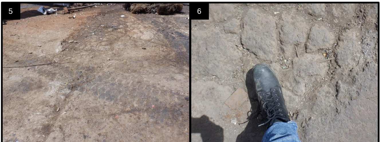
Photographs 5 & 6. Areas of damaged concrete impermeable surface.
