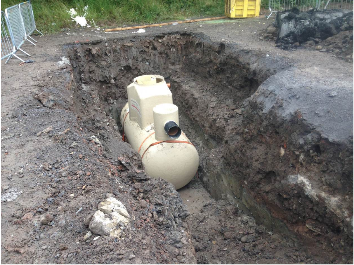
In-place oil interceptor
