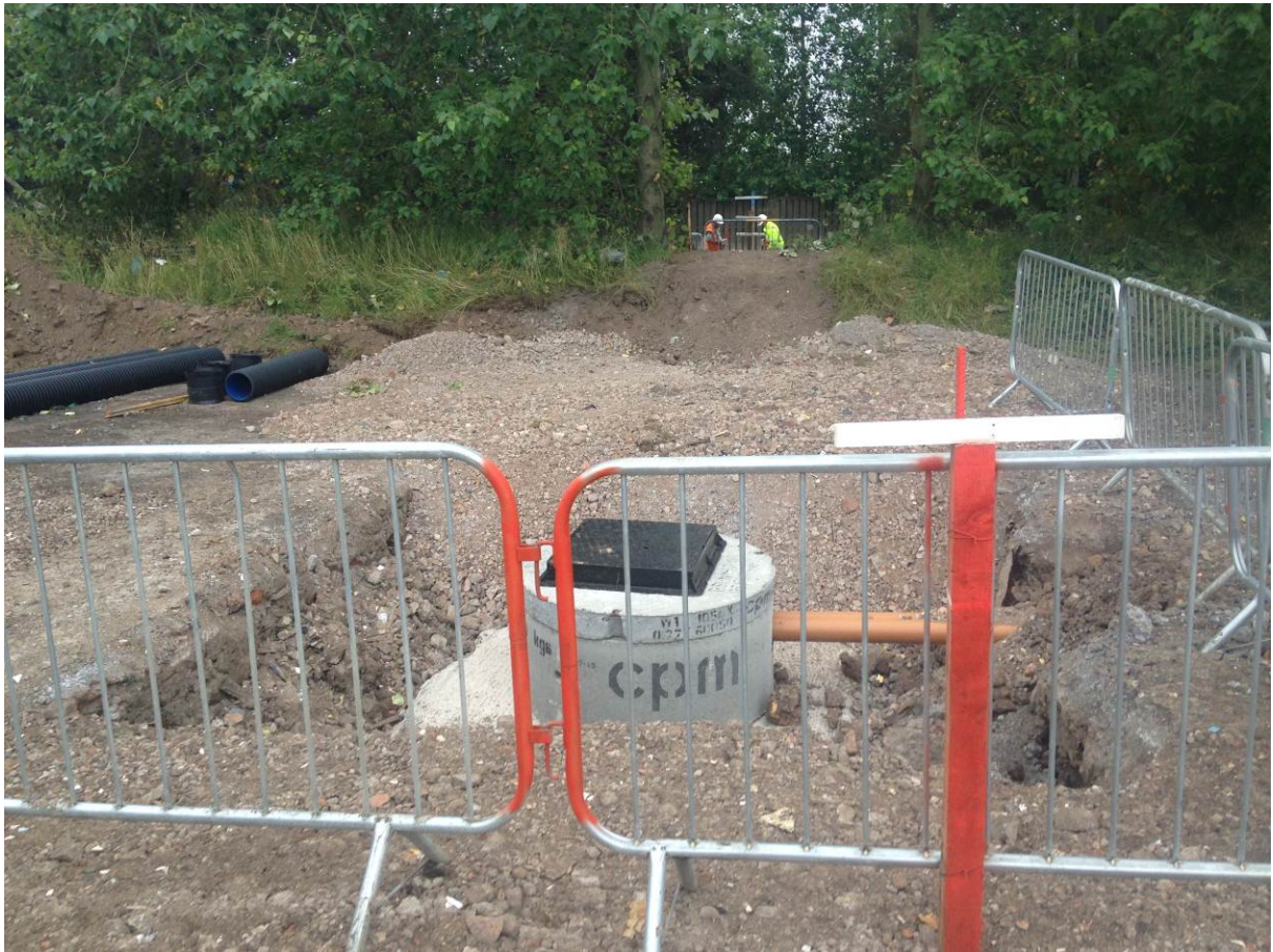
Oil interceptor access chamber
