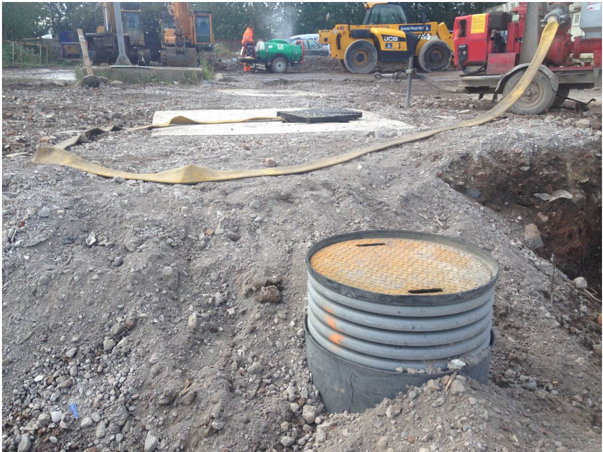
Shut-off valve chamber
