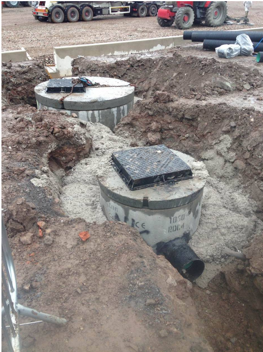
In-place silt trap (rear) and redundant chamber (front)
