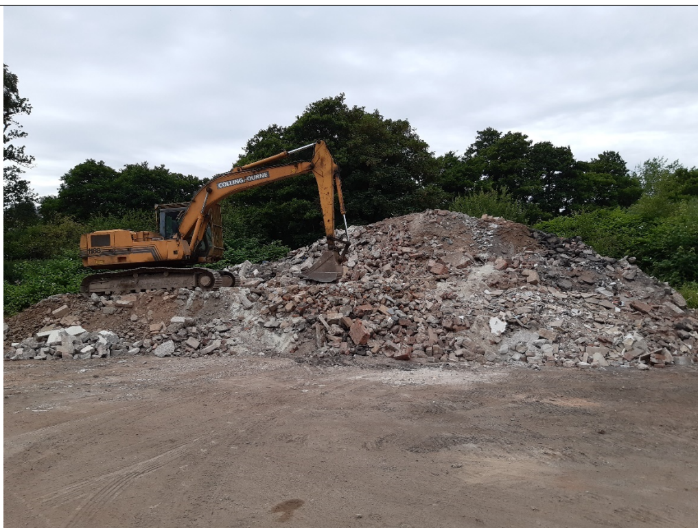
Photo 1 – waste stockpile consisting of wastes highlighted in red (below)
