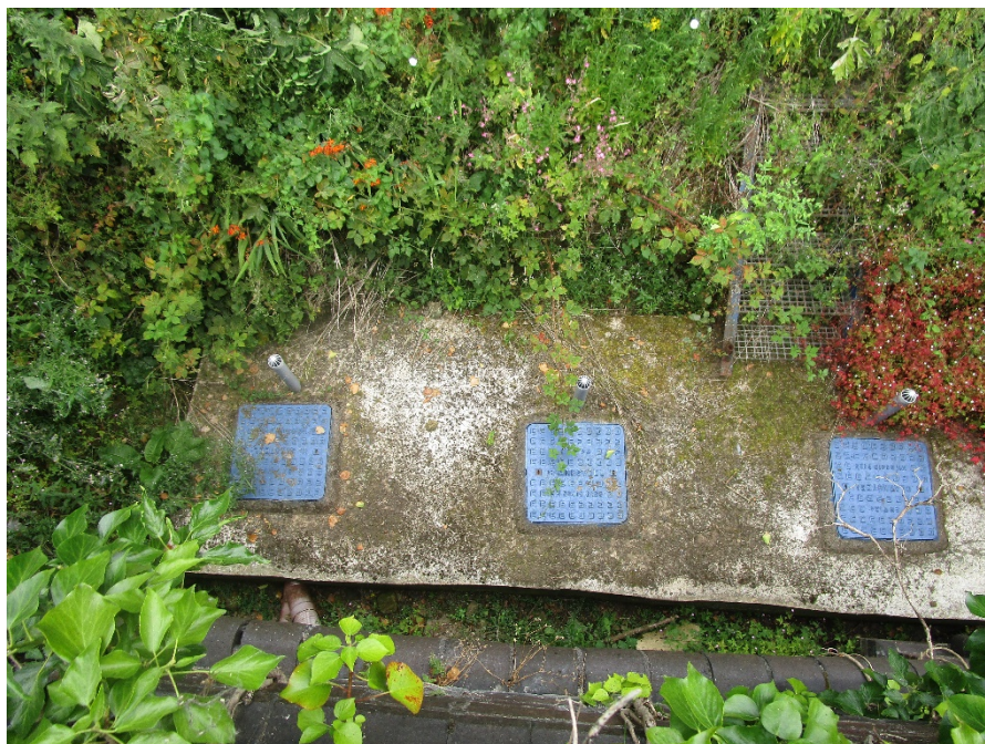
Figure 4. Oil interceptor for depollution yard drainage.
