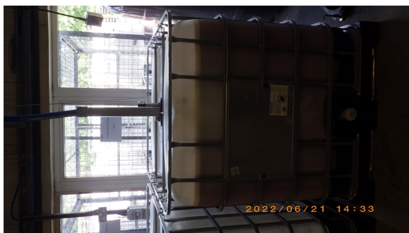
Photo of IBC which requires bund putting in place.
