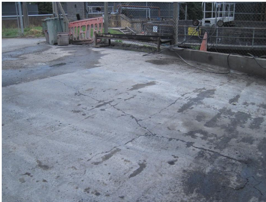
Photograph 3.2, View Of Cracking To The Surface Of The Concrete Base
