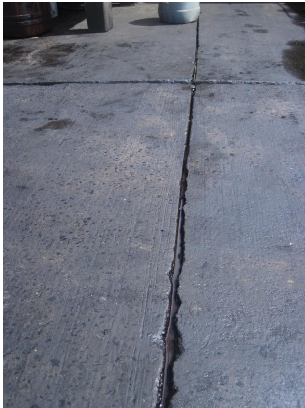
Photograph 1.4 Typical construction joint (showing missing sealant at surface)
