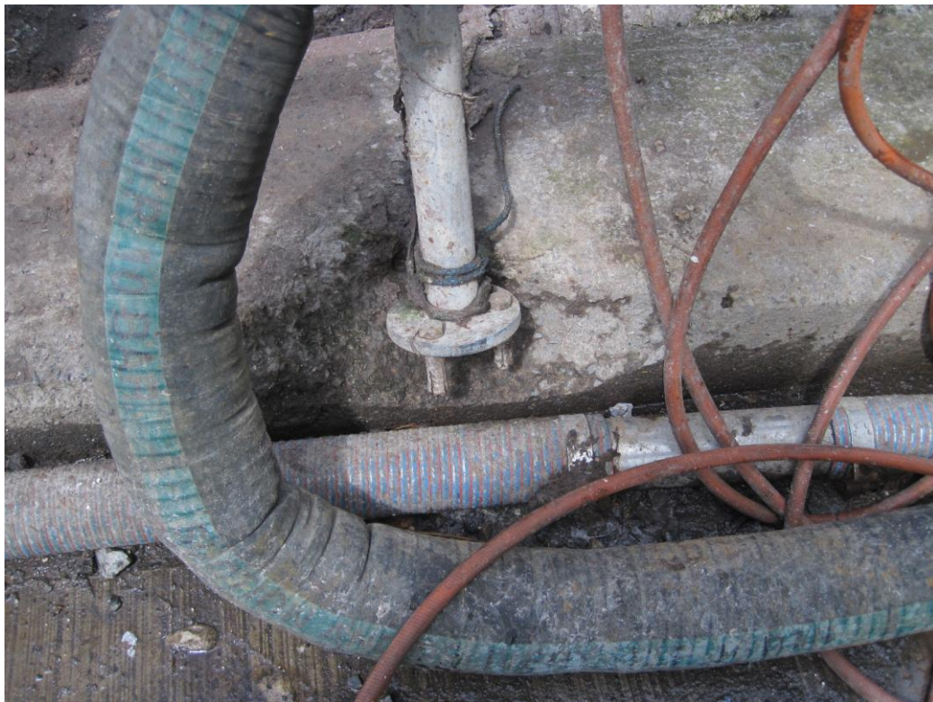
Photograph 4.2, Damage To Base Of Handrail Standard (North Bund Wall)
