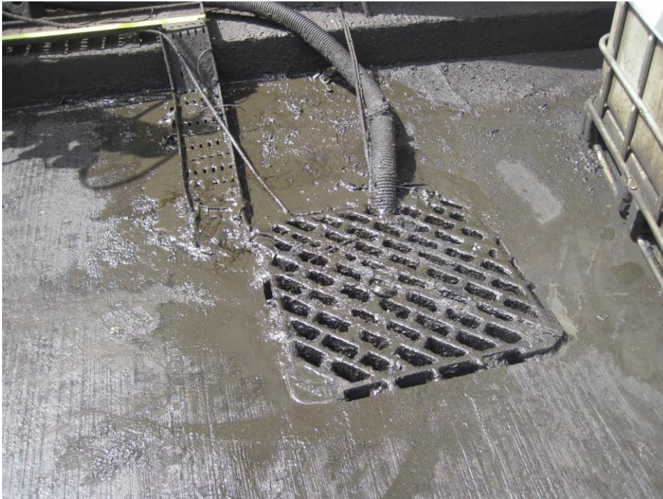
Photograph 1.5. View Of Gully At Dead Low Point Of Base
