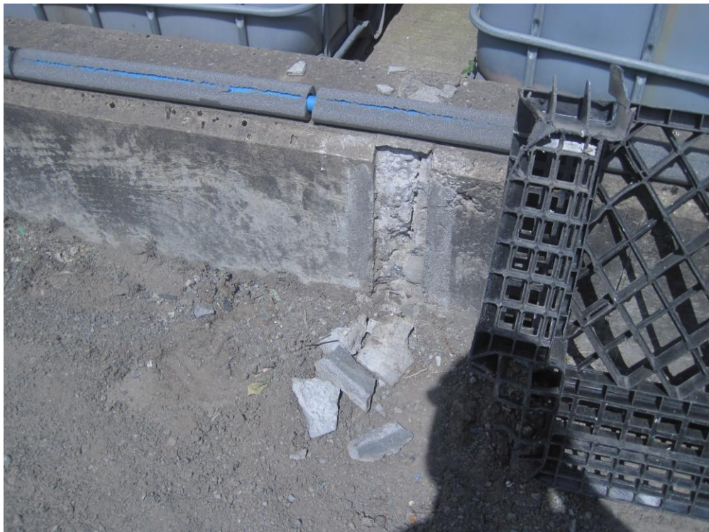
Photograph 1.13 View Of Spalling Of Concrete At Joint Location
