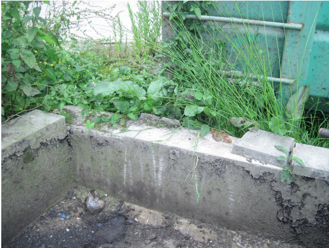
Phptograph 3.3, View Of Missing Coping To The Top Of The Wall
