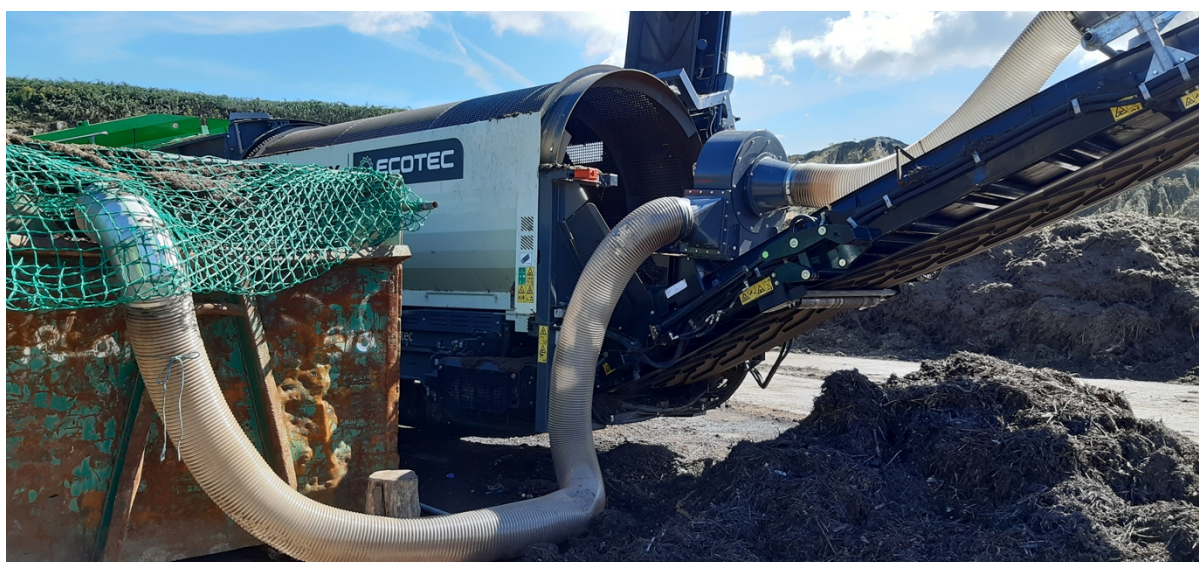
Photo 7 - Vacuum installed on composting treatment station
