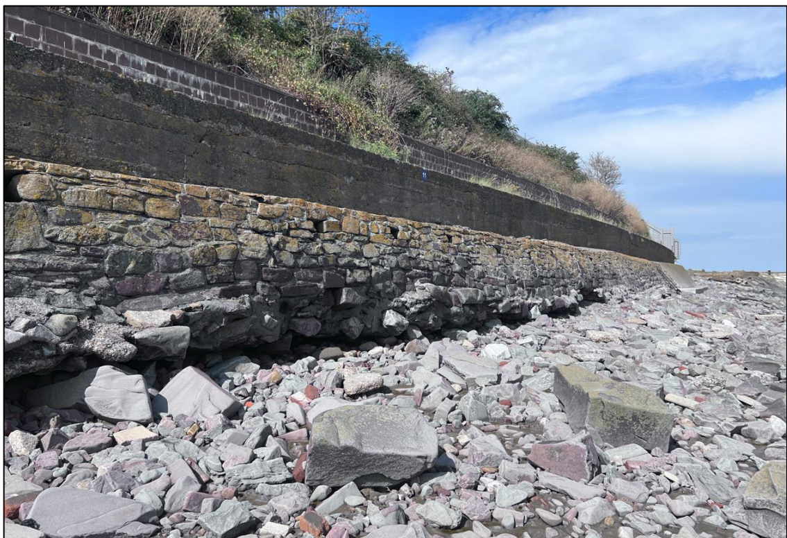
Figure 8: Significant scour failure below masonry toe of the structure further north.
