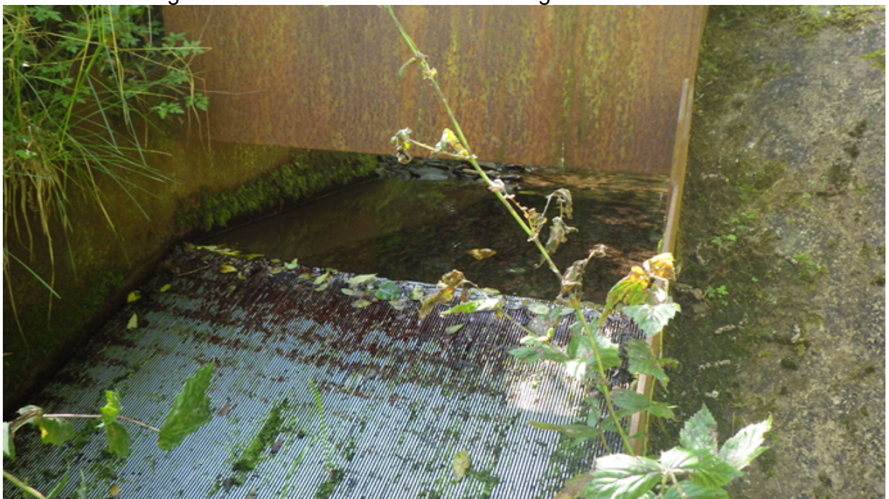
70/30% weir plate - incorrect flow split for this time of year
