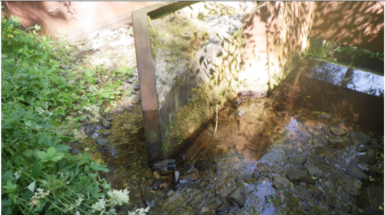
Water flow through screen box - incorrect flow due to gravel
