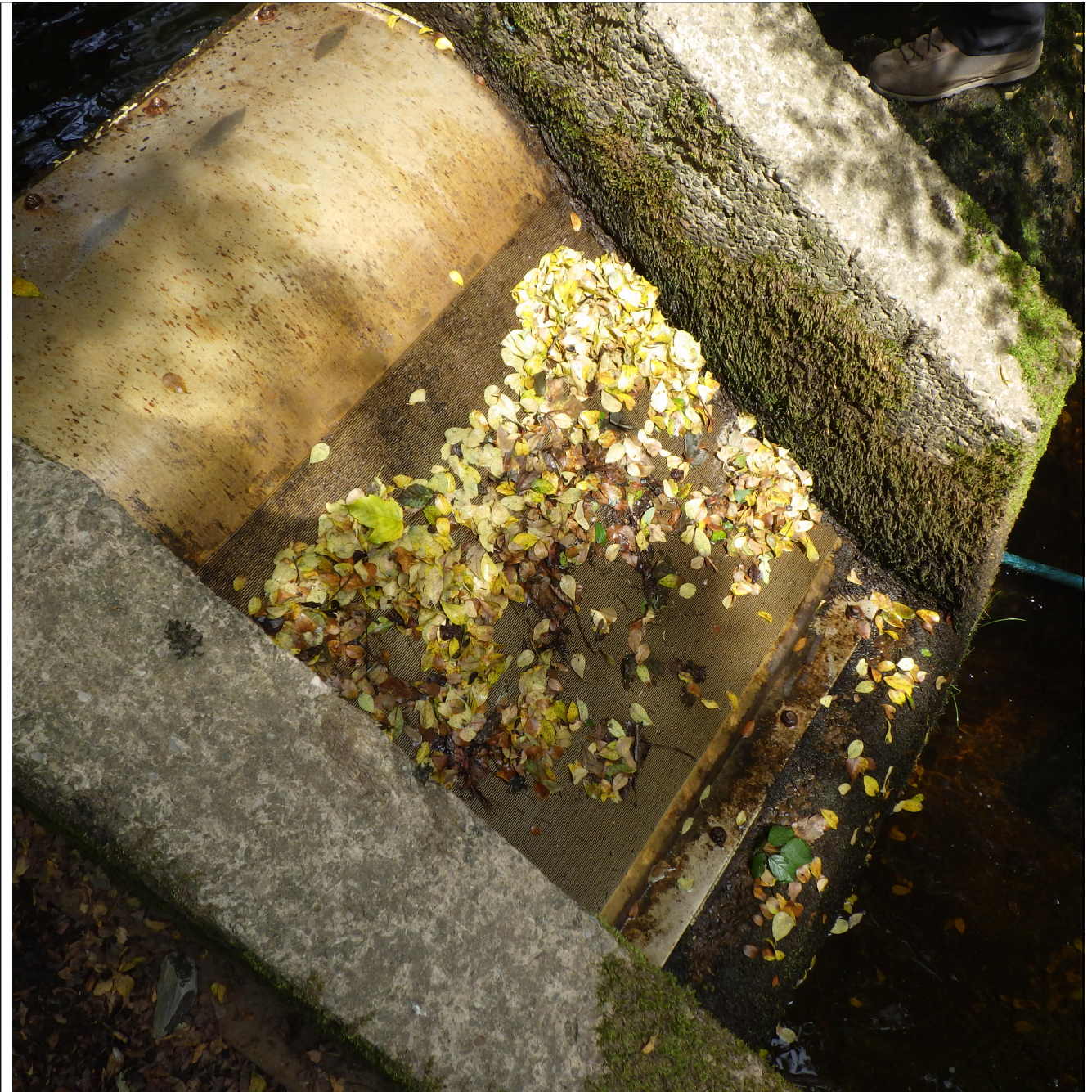
Blue pipe below impoundment
