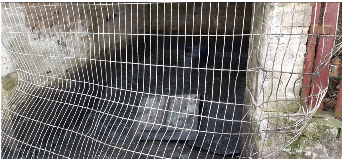
Photo 2 - Site interceptor working with no issues
