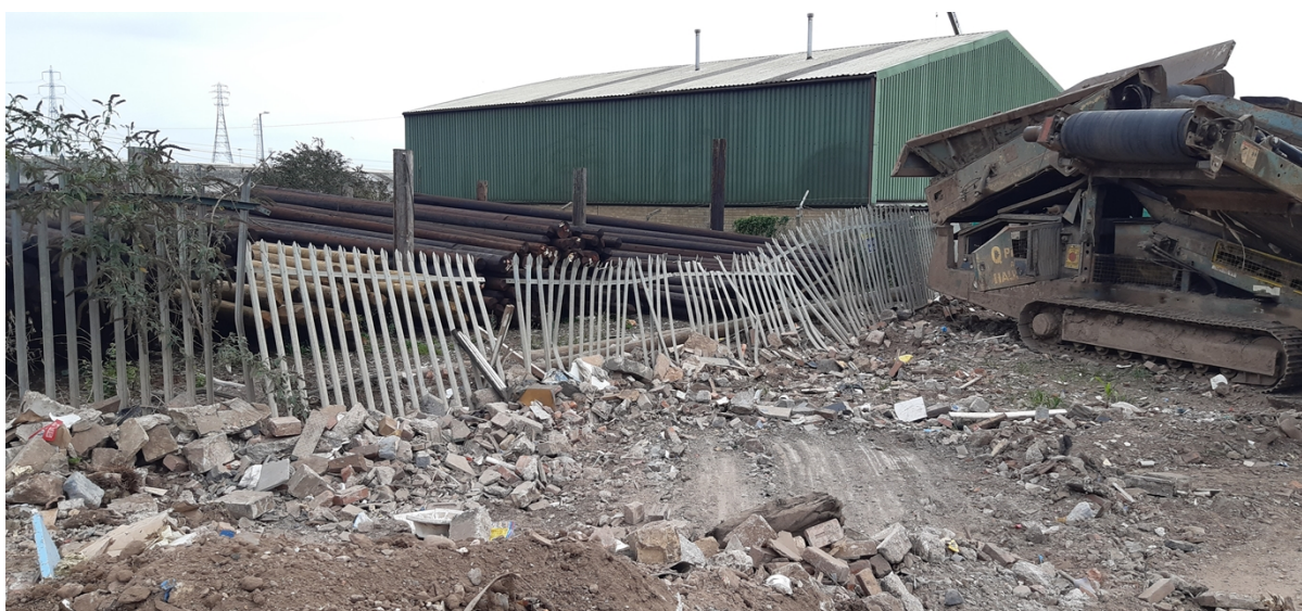
Photo 4 - Damaged security fencing at A1 Waste Management Ltd
