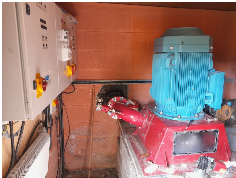
ED3 - Photo of Turbine
