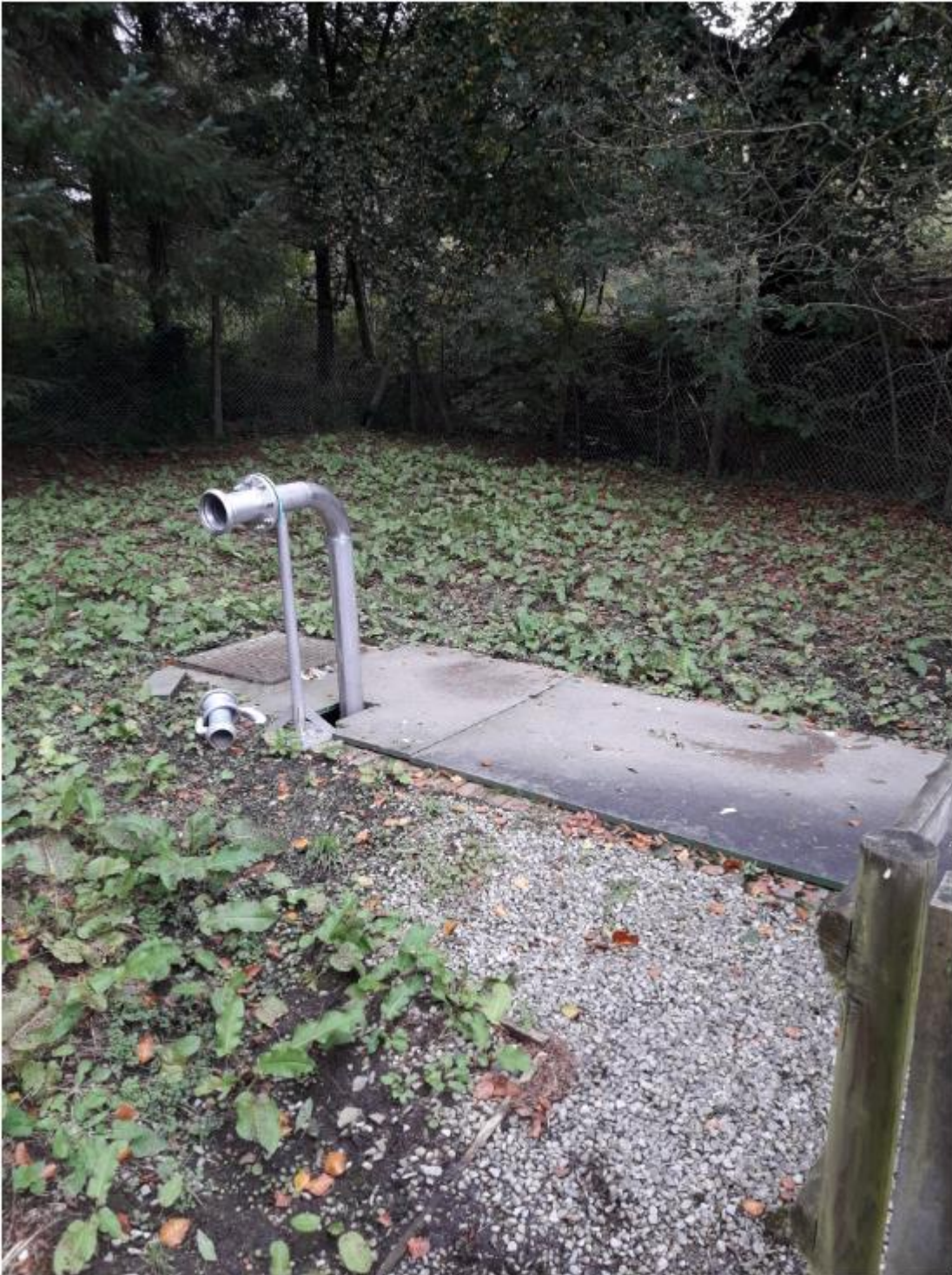
Inlet, primary tank and sludge tankering point.
