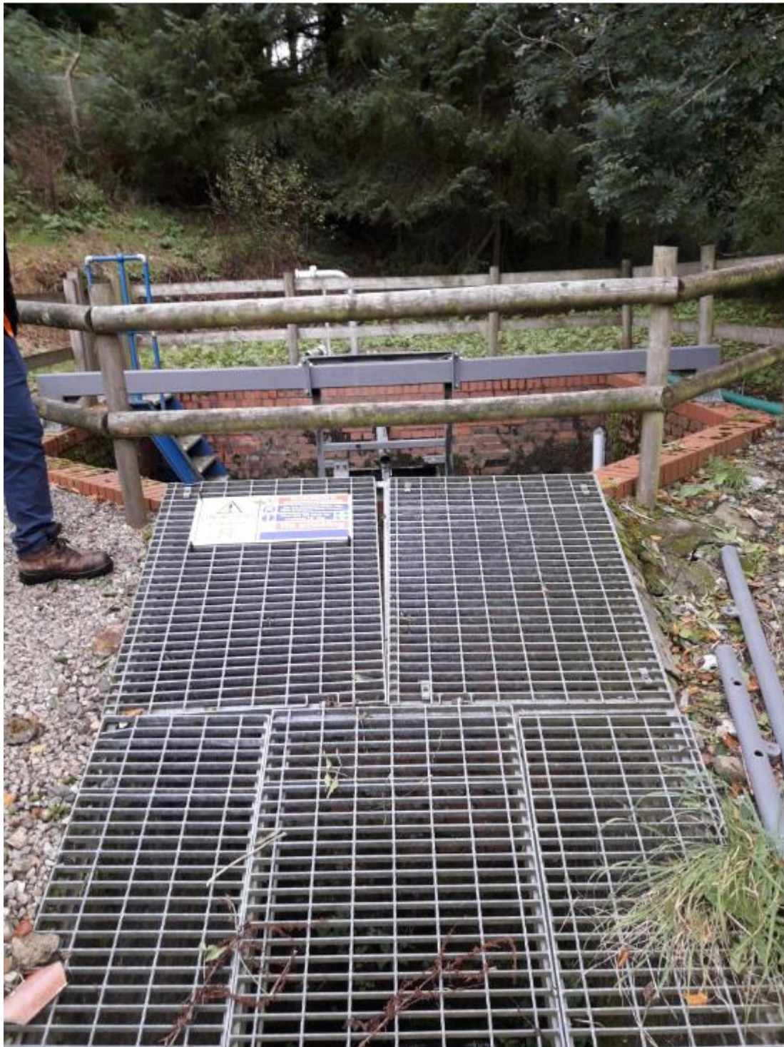
Outlet pipe from trickling filter bed flows into an open chamber where it can be observed.
