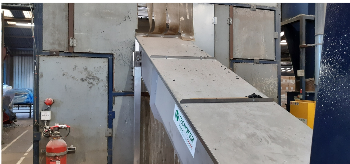
Photo 6 - Enclosed conveyor belts to reduce noise and improve housekeeping
