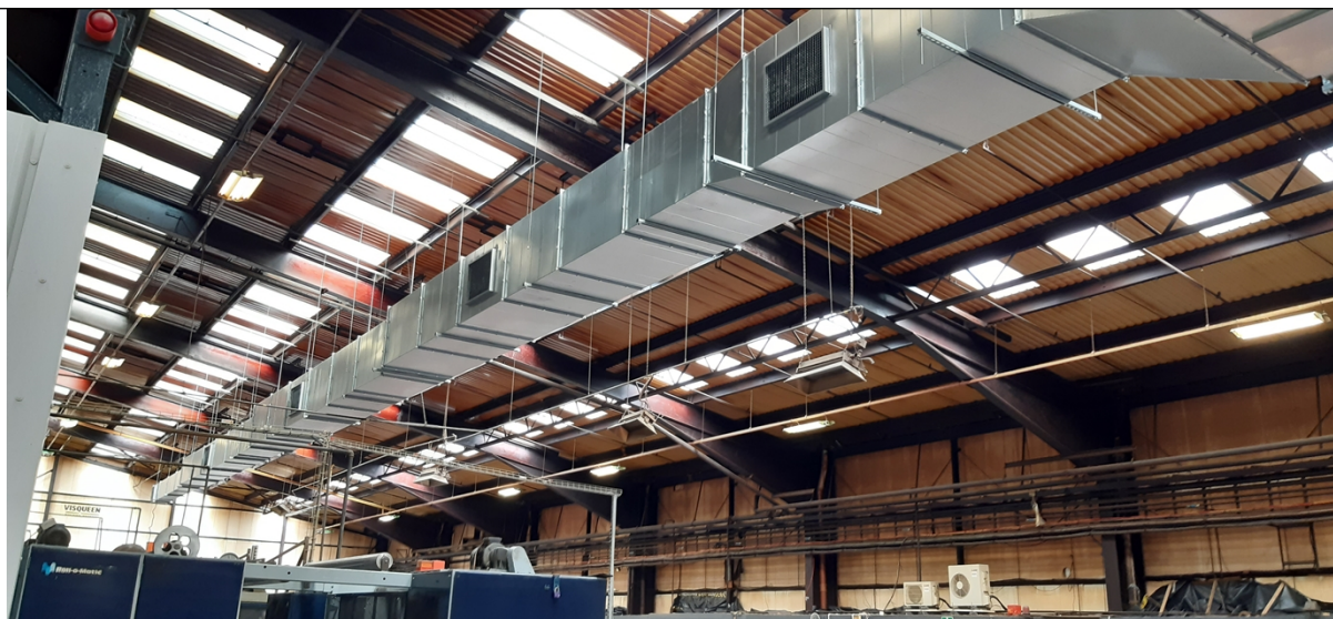
Photo 7 - Newly installed Air Handling Unit (AHU)
