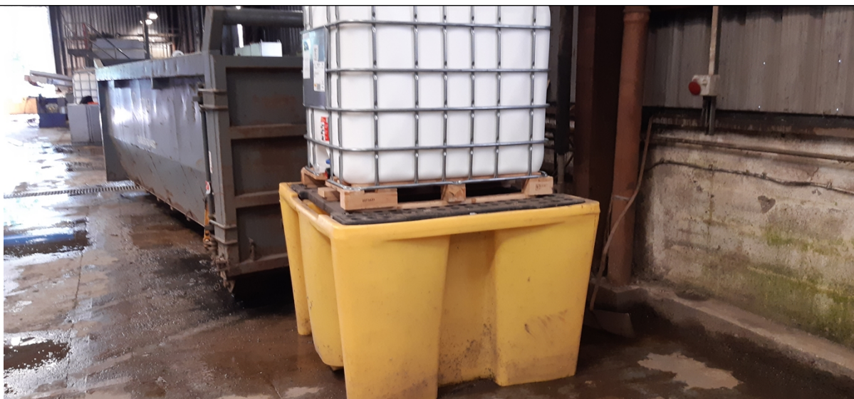
Photo 5 - Secondary containment bund for liquid storage
