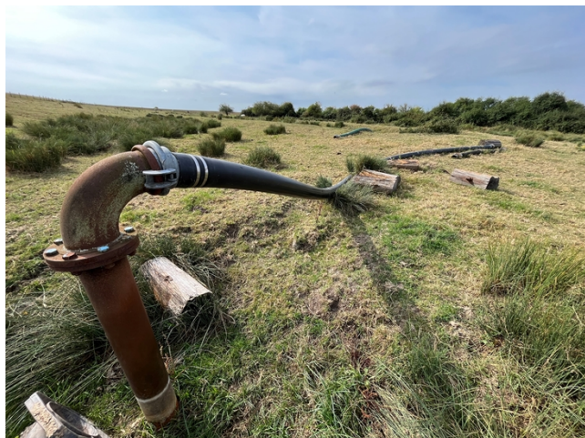
Photograph 2: Disconnected pipework at abstraction point B.
