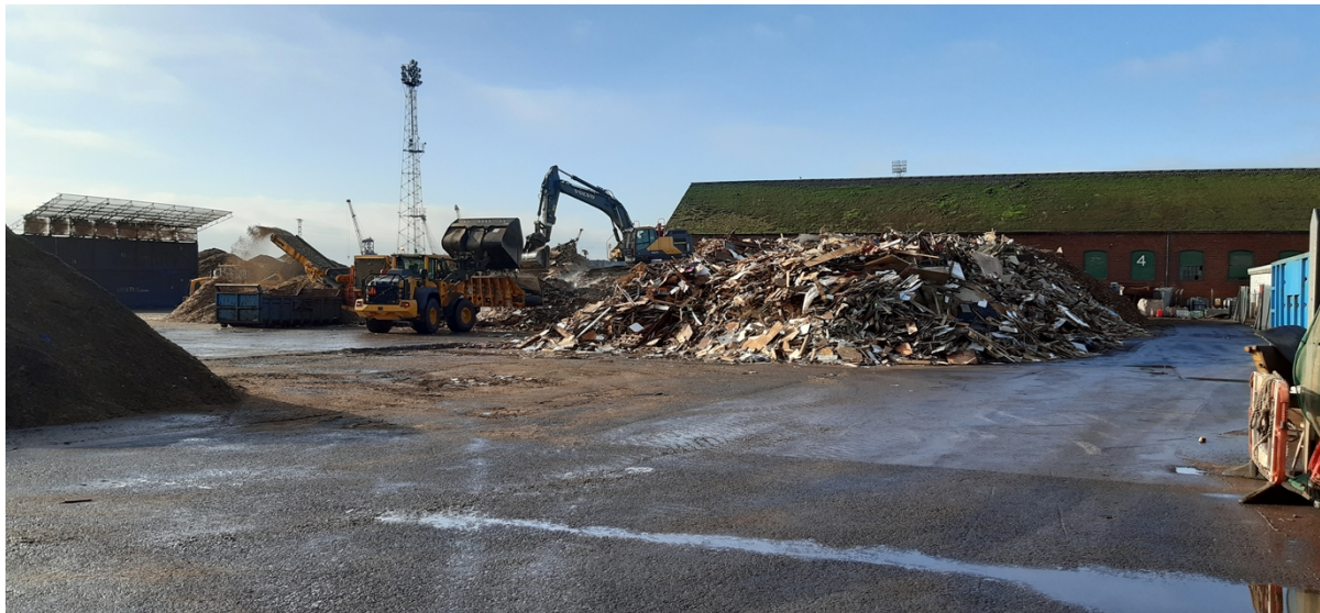
Photo 1 - General housekeeping on site was of a good standard
