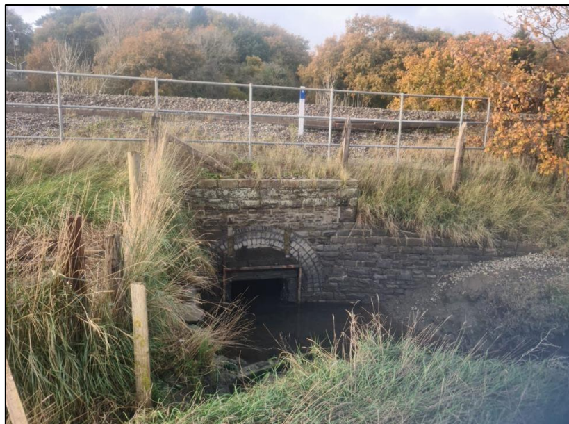
Figure 2: Damaged tidal flap.
